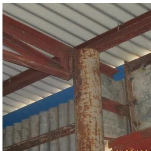
Truss were poorly welded with steel pipe column in Grey fabric store
