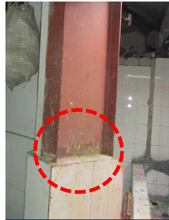
Corrosion was observed on steel column in 1 st floor's printing section
