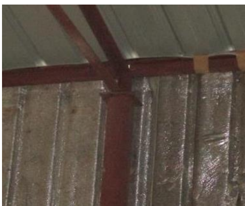
Truss were poorly welded with steel pipe column in Jhut store
