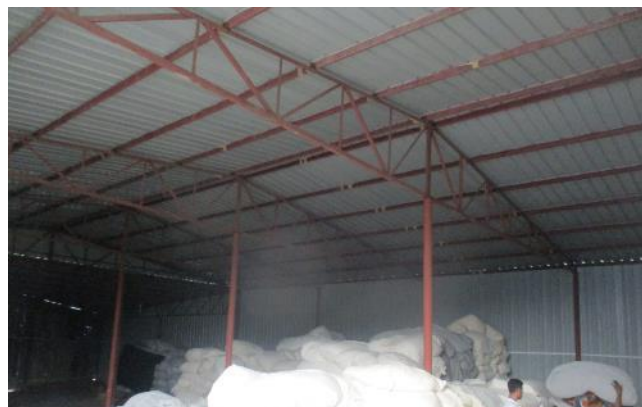
Typical truss frame with out any horizontal or vertical bracing system in Jhut store
