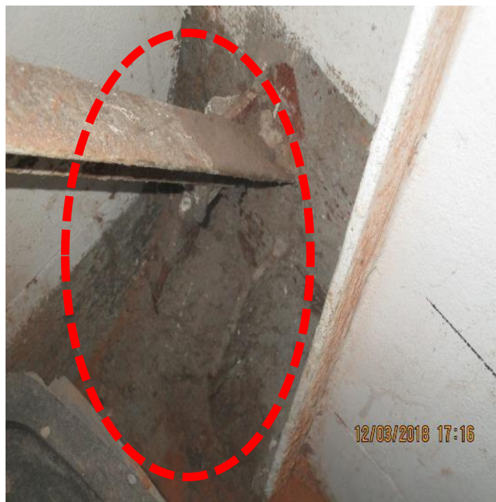
Corrosion was observed at joint of angle bracing and column in ground floor
