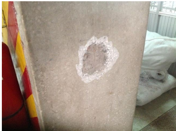
Tested Basement Column 8 Storey Building – Stone Chips
