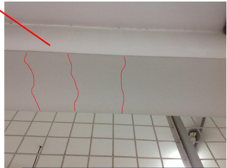
Cracking in beam supporting 2 nd floor
