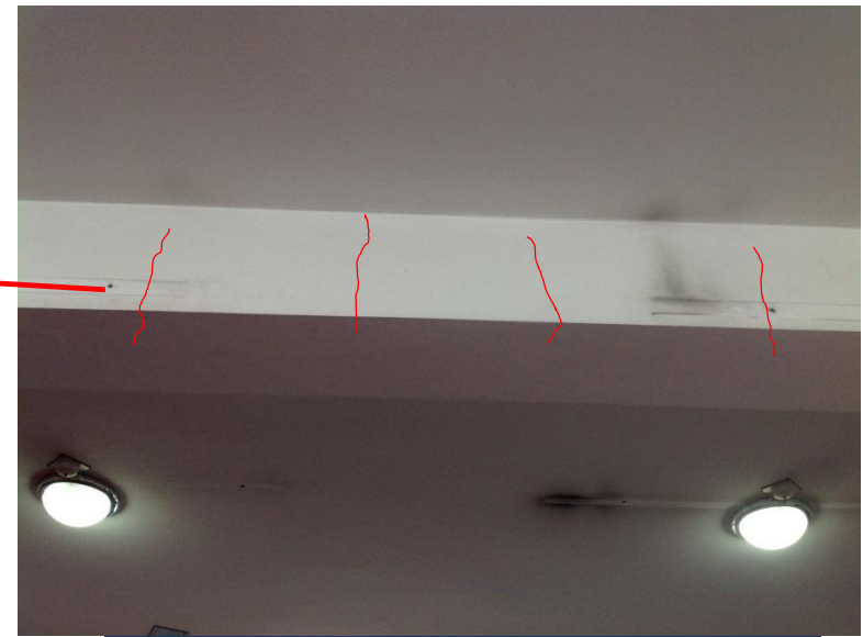
Cracking in beam supporting 5 th floor
