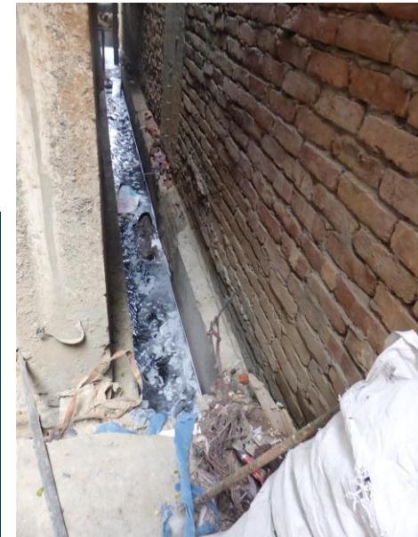
Many open drains, gulleys and large excavations throughout the factory complex – both within and around buildings.
