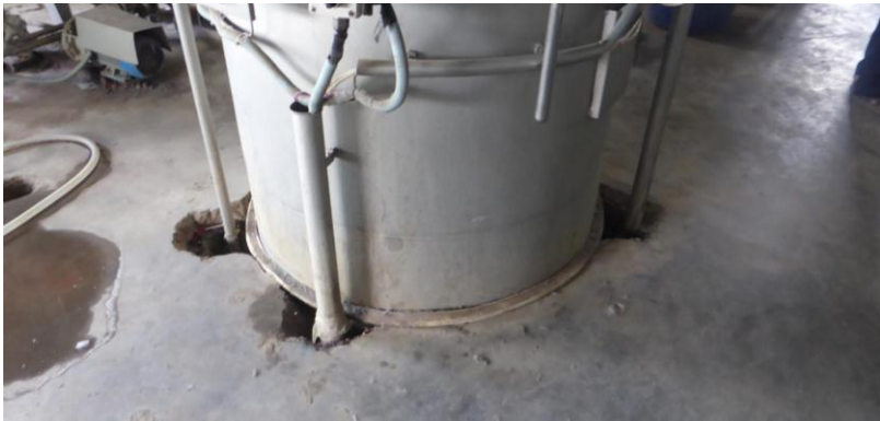
Numerous undocumented openings within Building 5 mezzanine slab.
