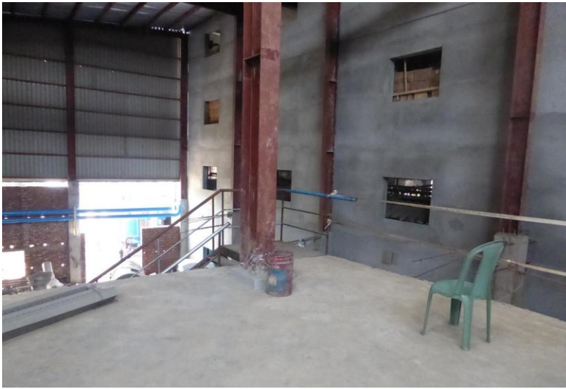
Unprotected open edges at mezzanine level in Building 5.
