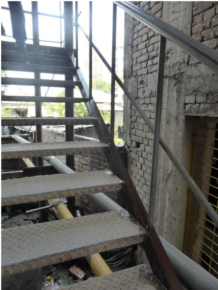
Some evidence of minor corrosion to steelwork. Water flowing down stairs between Building 3 and Building 6.
