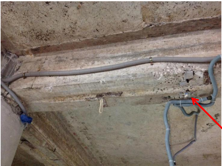
Rough finish to concrete – slab soffits, beams and columns. Rust staining on soffits.
