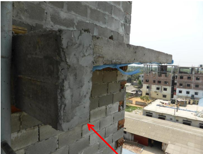
Workmanship issues with concrete
