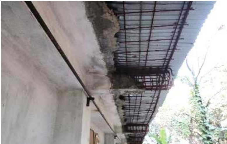
Exposed rebar on 1 st floor slab
