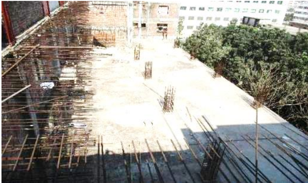
Exposed rebar on column and slab
