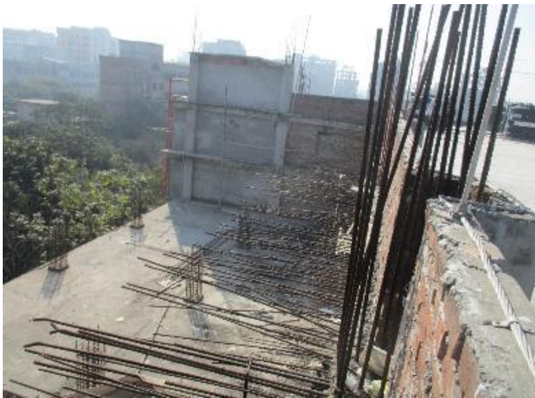
Exposed rebar on roof
