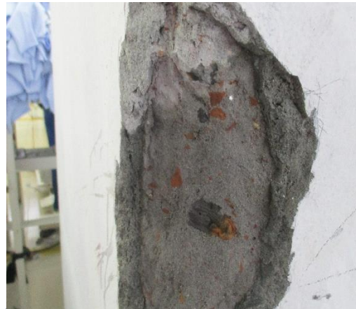
Brick chips aggregate at existing column
