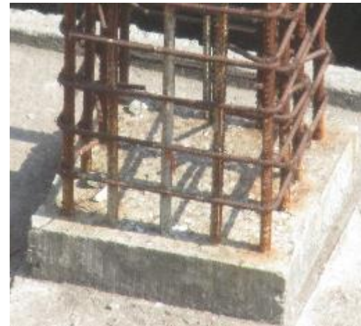
Corrosion observed on exposed rebar
