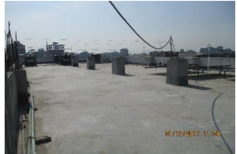
No obvious drainage system was observed
