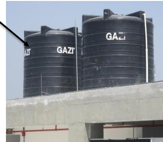
Two nos. 10000 liter water tank on stair case roof slab
