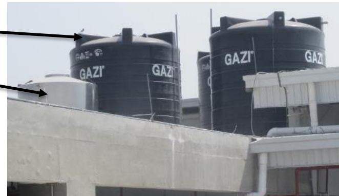
Three nos. 10000 liter and single 5000 liter water tank on stair case roof slab
