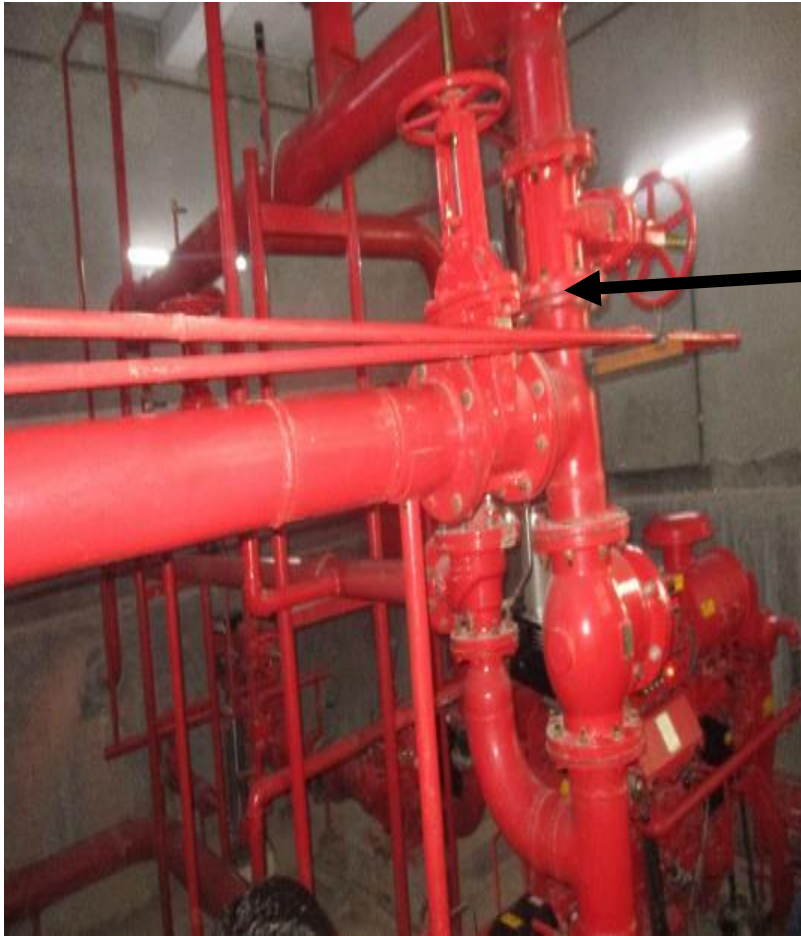
Pump Room below Ground Floor
