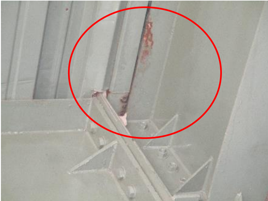
Corrosion observed at main beam under deck slab.
