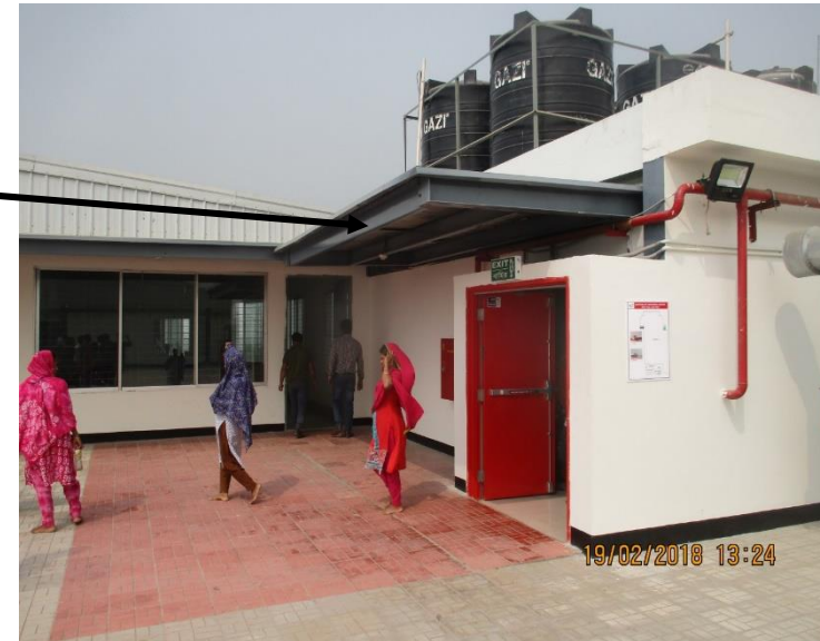
Extended canopy in front of the stair case did not shown in drawing
