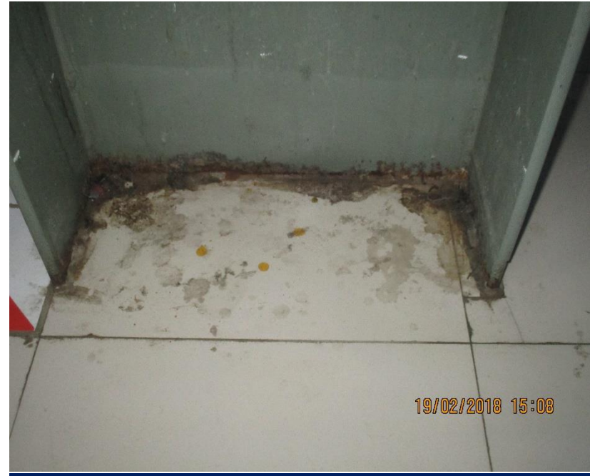
Corrosion was observed at joint of deck slab and steel column of 2nd floor production areas.
