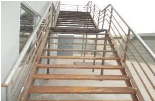
Corrosion observed on the stair
