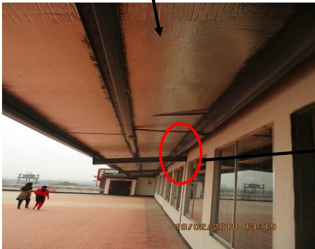
Extended beam of roof top shed was shown as CR-201 section but detail of the beam was not available
