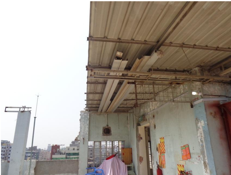
Poorly Framed Steel Canopies
