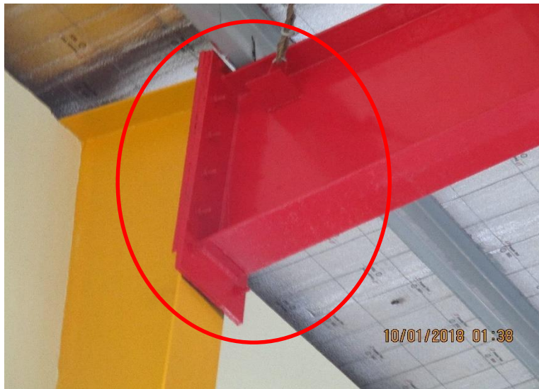
Existence of significant gap at connection
