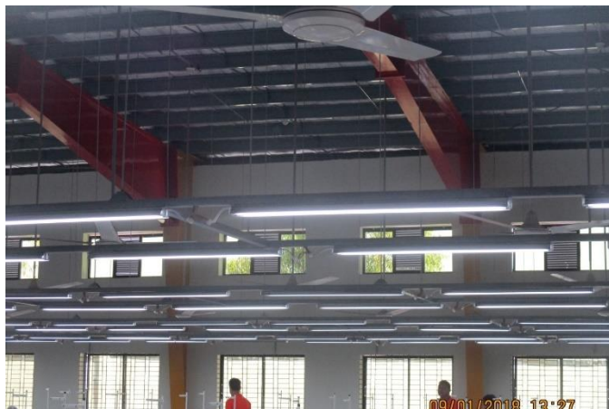
Missing strut member in eave level
