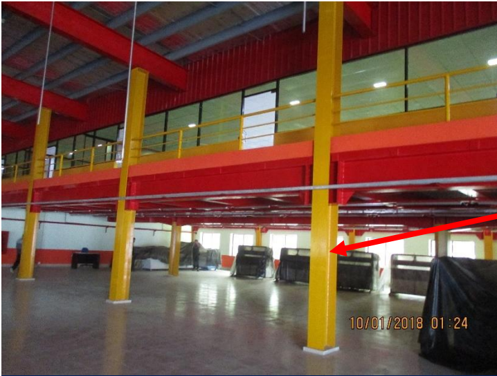
Column extended up to rafter with pin head not shown on drawing.
