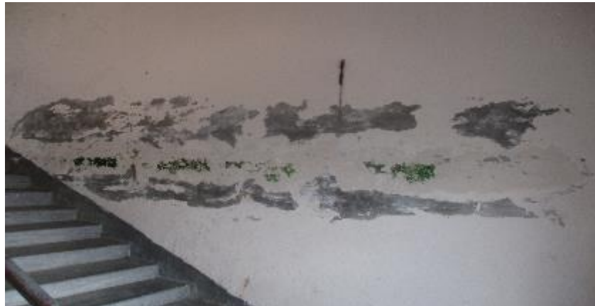
Dampness on wall between stair and toilet portion
