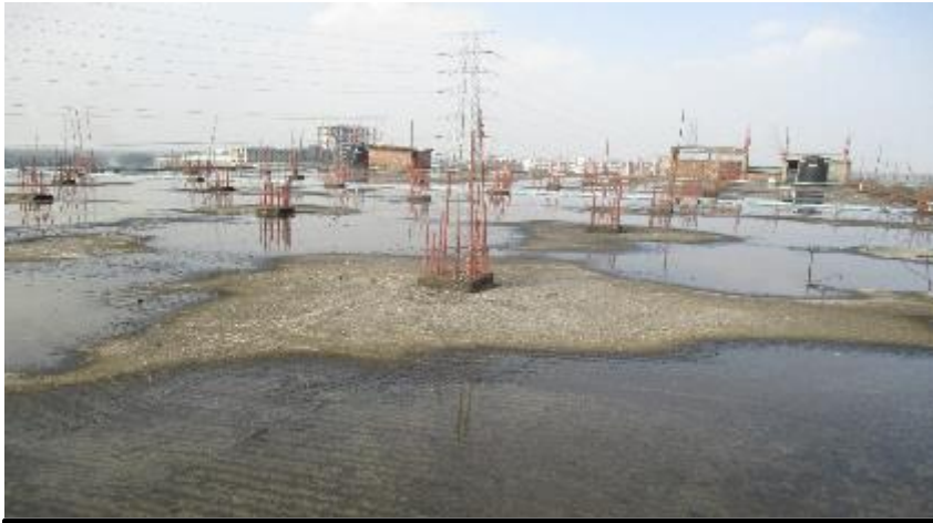
Water ponding on roof
