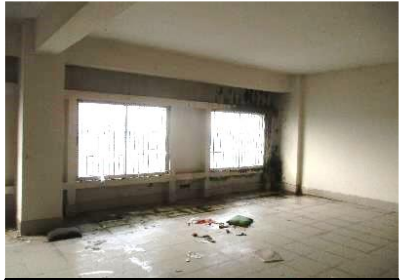
Dampness on wall at inner façade wall
