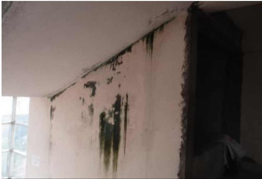
Dampness on wall at lift core portion
