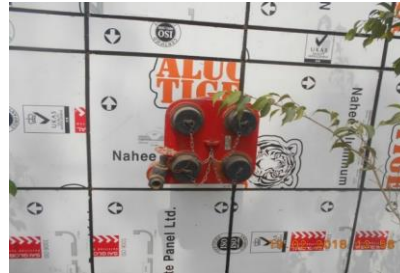
Fire Department Connection
