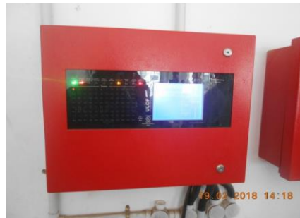
Fire Alarm Control Panel
