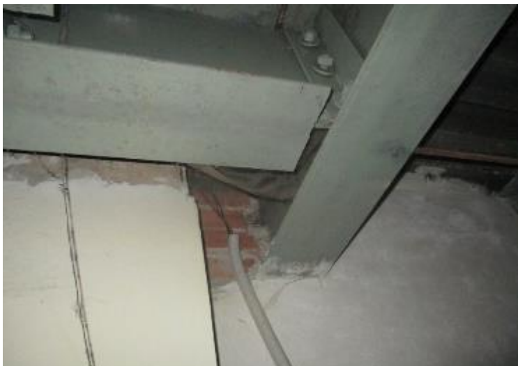
Loose nuts on some bolted joints
