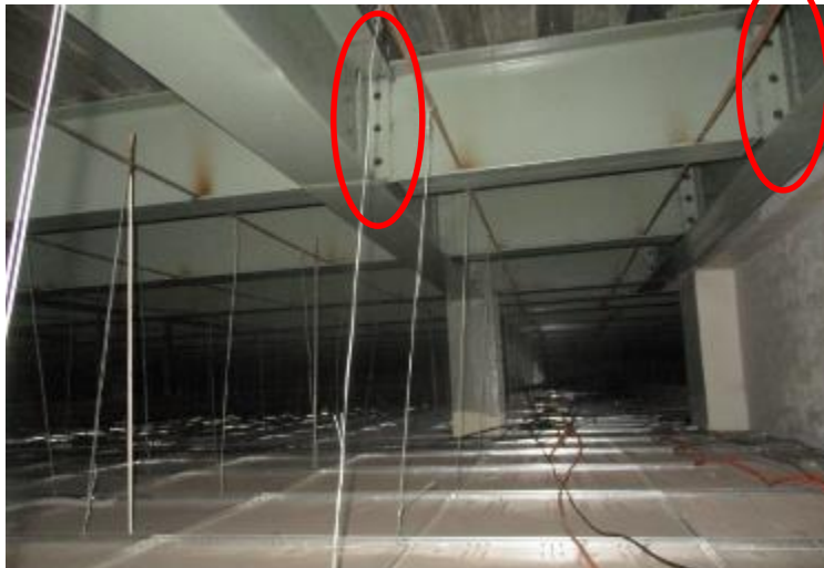
Welded joints instead of bolt joints
