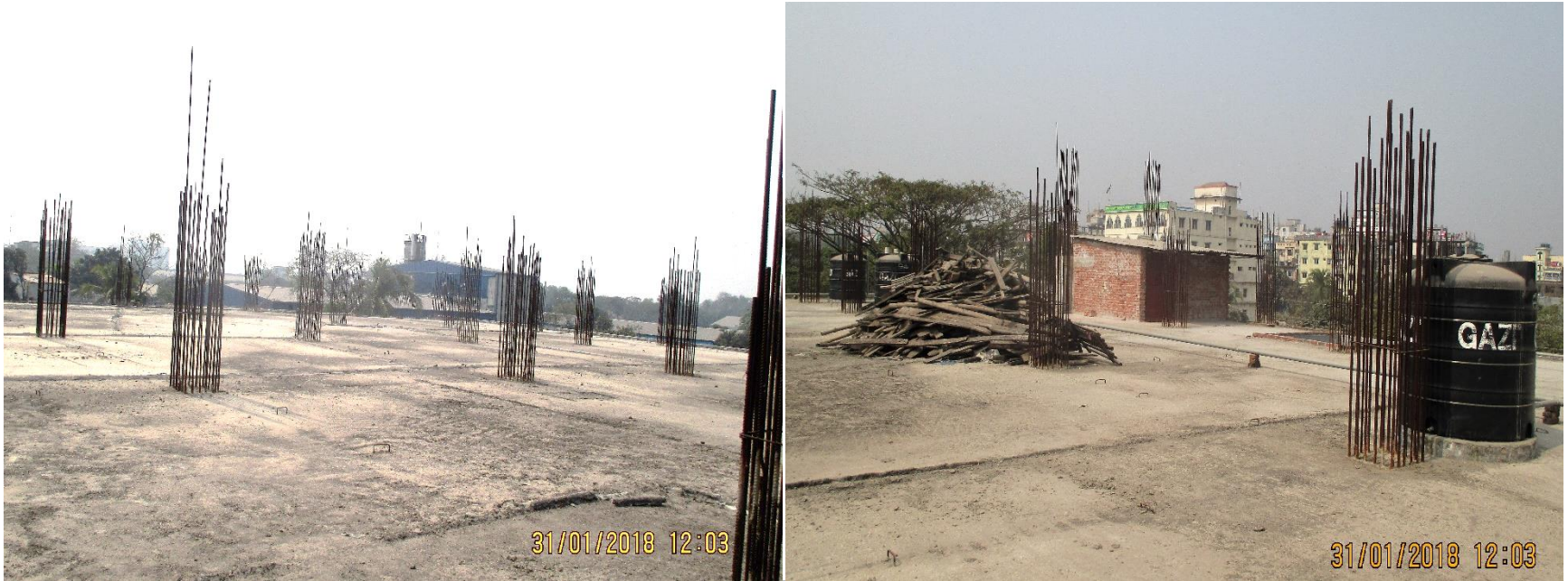
Rebar exposed to weather
