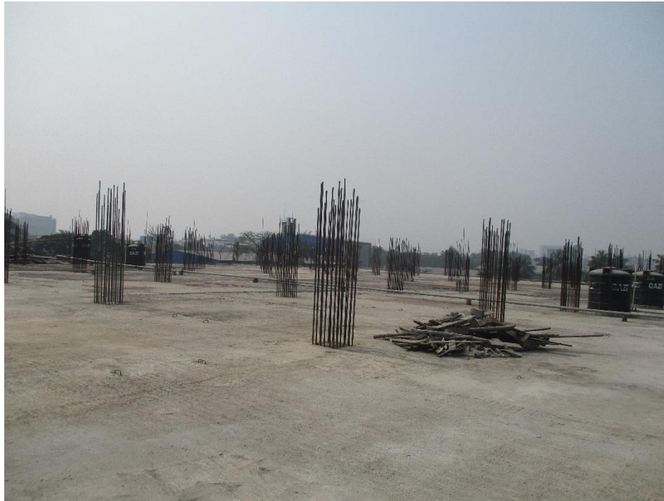
Exposed rebar on roof indication of future extension
