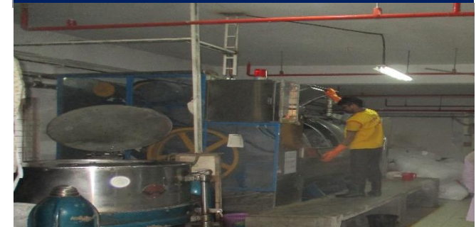
Dryer machine with build up at ground floor
