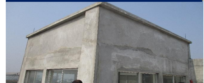
Water tank at roof
