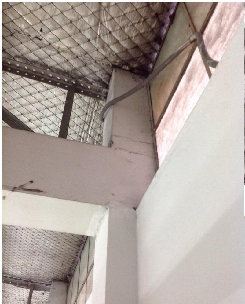
Cracking at Connection of Lightweight Roof
