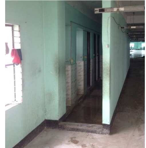
Typical toilet block
