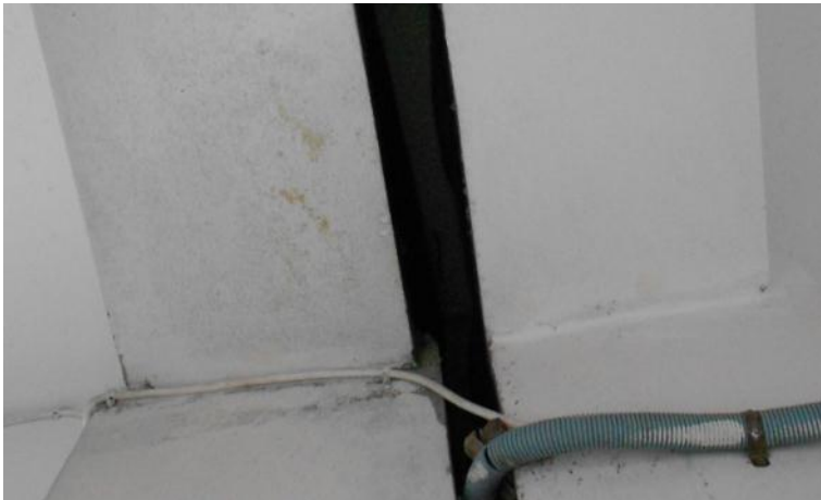
Water causing damage and possible corrosion
