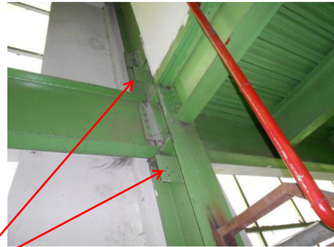
Missing X bracing along GL1 – cleat plates present
