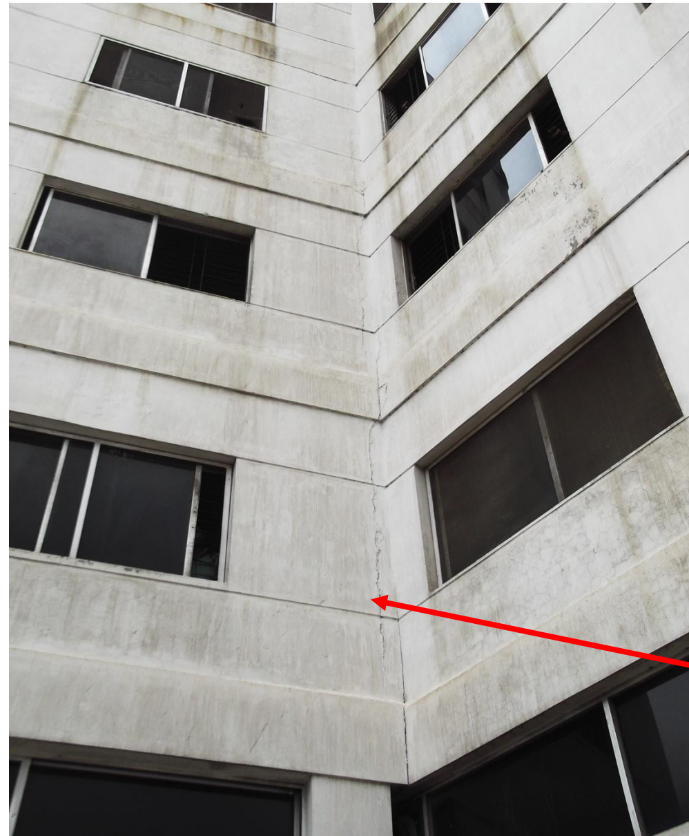
Cracking at Interface Between Main Building and 5 Storey Annex
