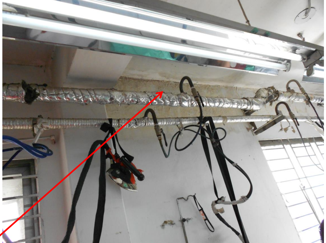
Water damage due to condensation from ironing
