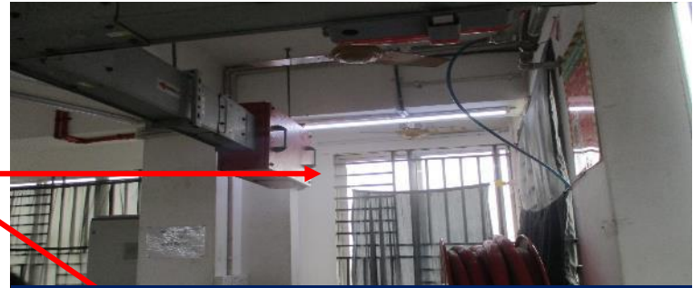
The marked cantilever on south side was not mentioned in as built drawing
