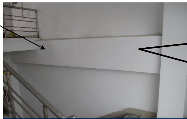
B-4 type beam on staircase was measured 625mm instead of 500mm
