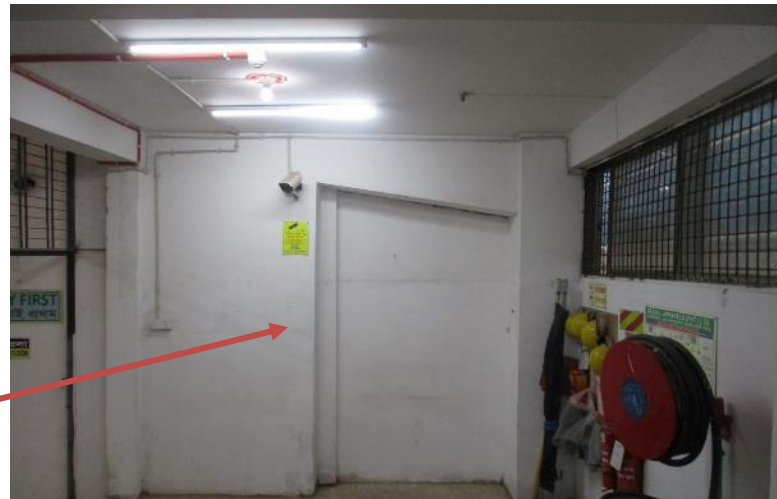
No core wall was found around the lift, only L-shaped column found
