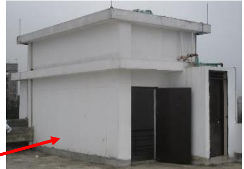
Water tank (4.9mx2.4mx1m)
