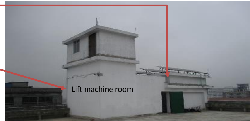
Height of the lift machine room was measured 6.5m instead of 4m. Also, the over head water tank height was measured 1m in place of 1.6m
