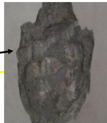
Stone chips aggregate found in basement floor column
