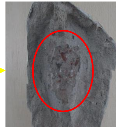
Brick chips aggregate found in 1 st floor column
