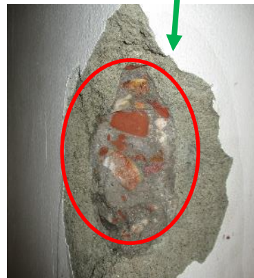
Mixed of stone and brick aggregate found in ground floor column
