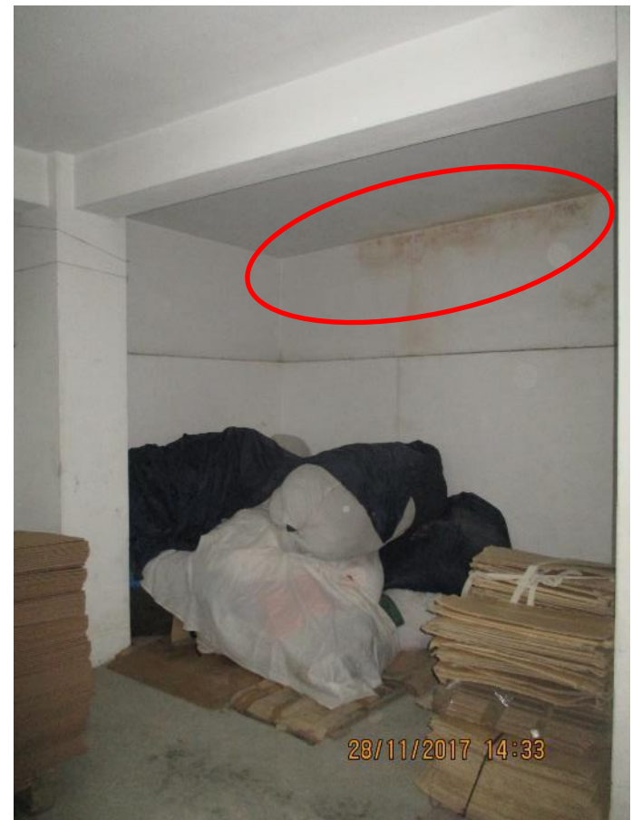
Dampness was observed on South West corner of basement wall
