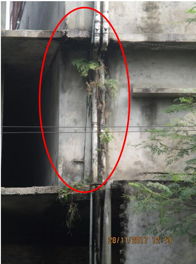
Vegetation was observed on west side facade wall
