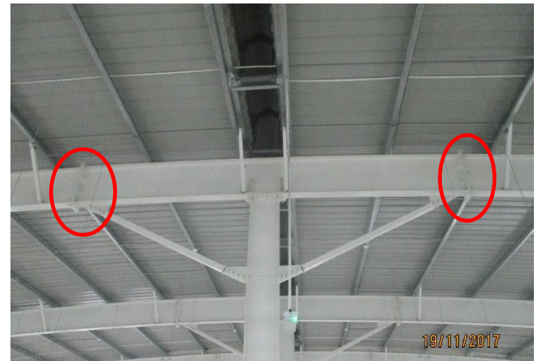
Additional joints in rafter were not shown in drawing
