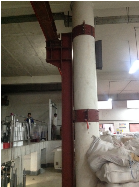
Crane beams attached to a number of columns in Building 4 applying additional loading.
