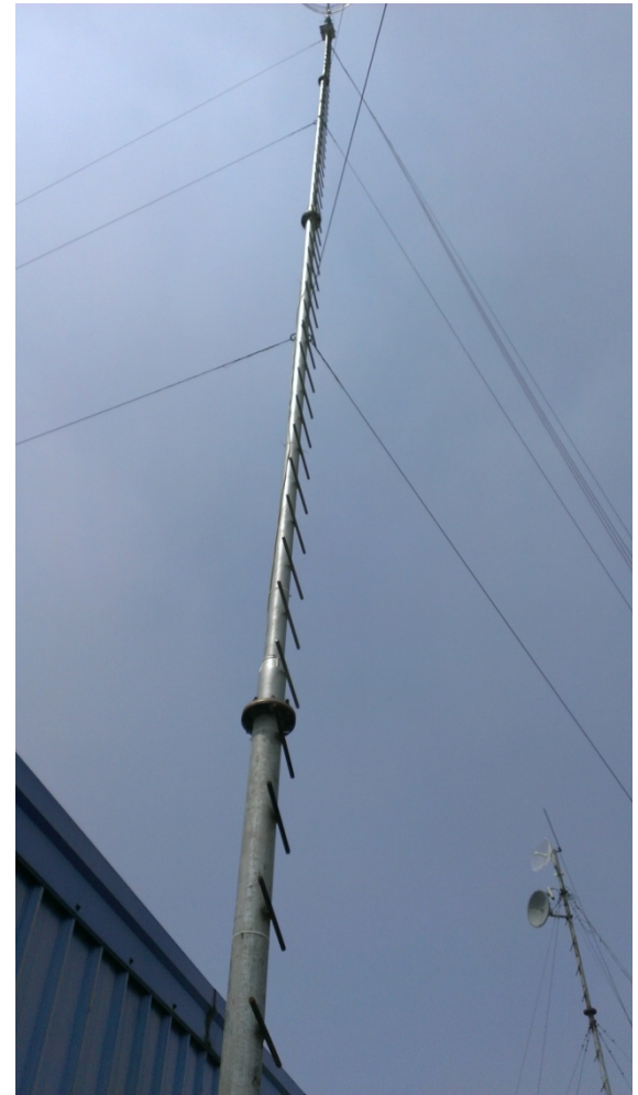
Communications mast supported on structure on roof of Building 1- Horizontal and vertical loads.
