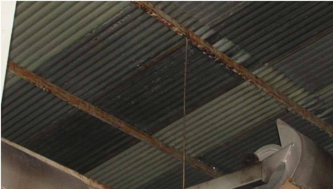
Rusting on steel shed member
