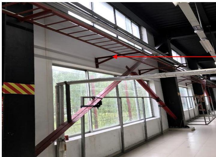
Bracing not continued to the column
