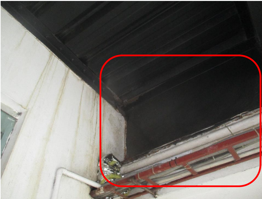
Corrosion at beam-column joint
