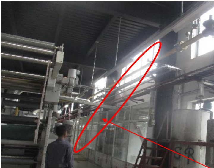
Bracing missing at one direction
