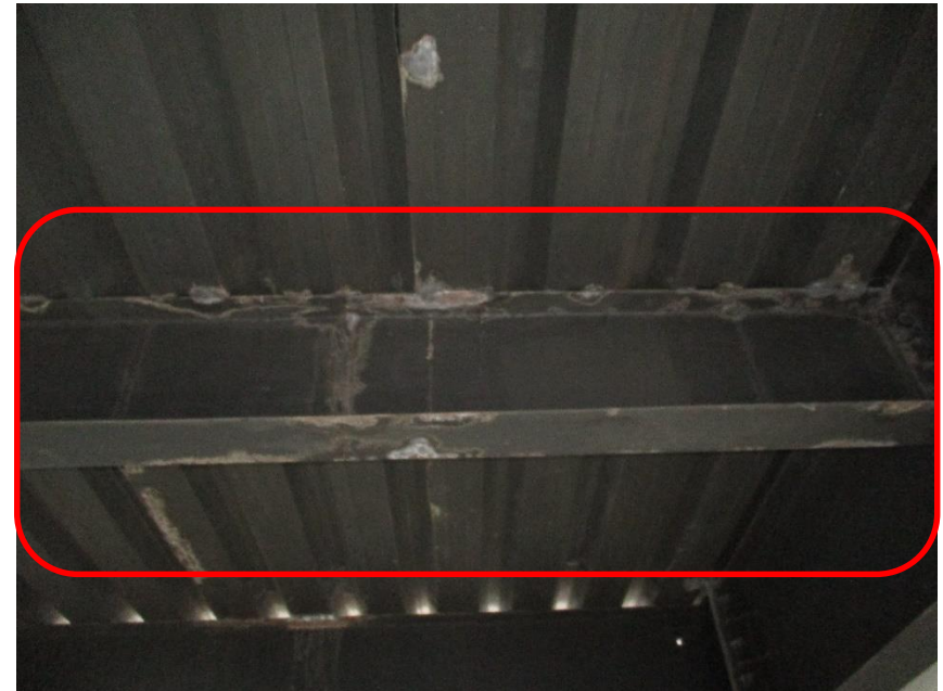
Corrosion at beam-column joint
