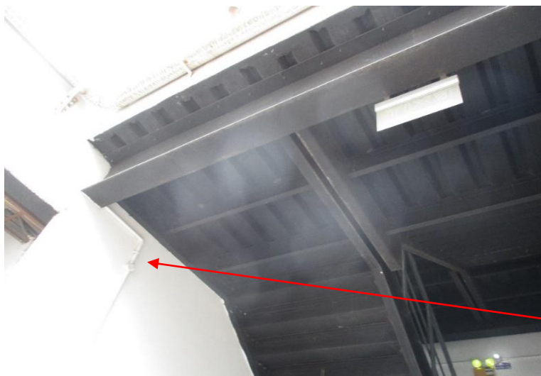
Bracing missing at stair -1
