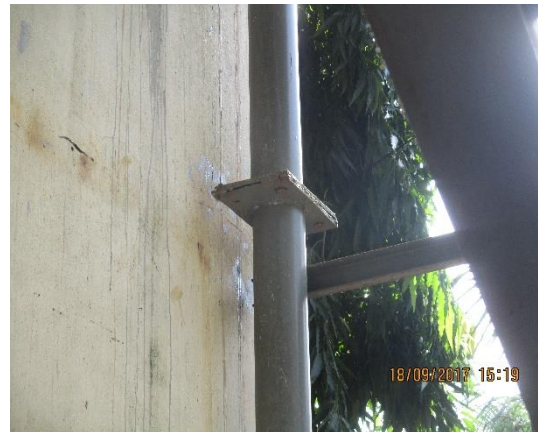
Weak joint of the pipe column due to poor welding
