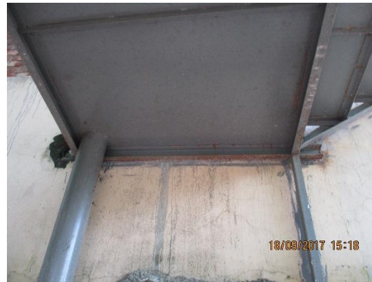
Weak support due to undersize steel box
