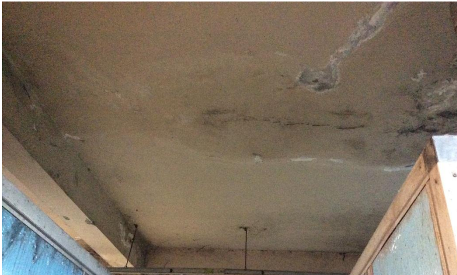
Shed 1 – Water damage to roof slab
