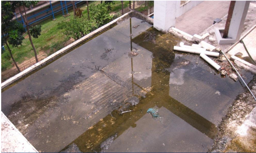
Ponding to roof slab
