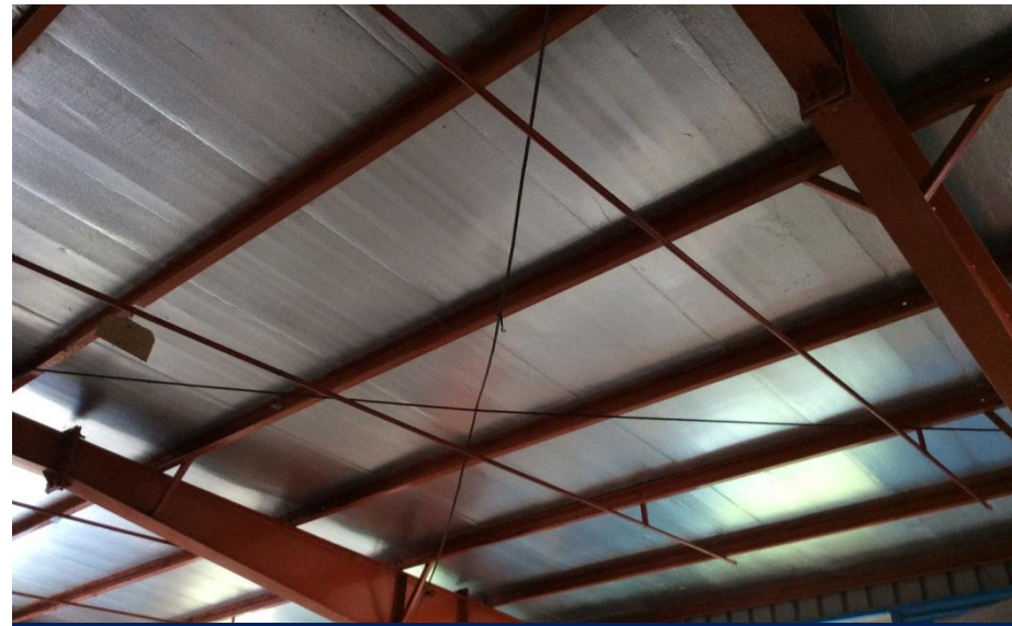
Shed 5 – Loose Bracing
