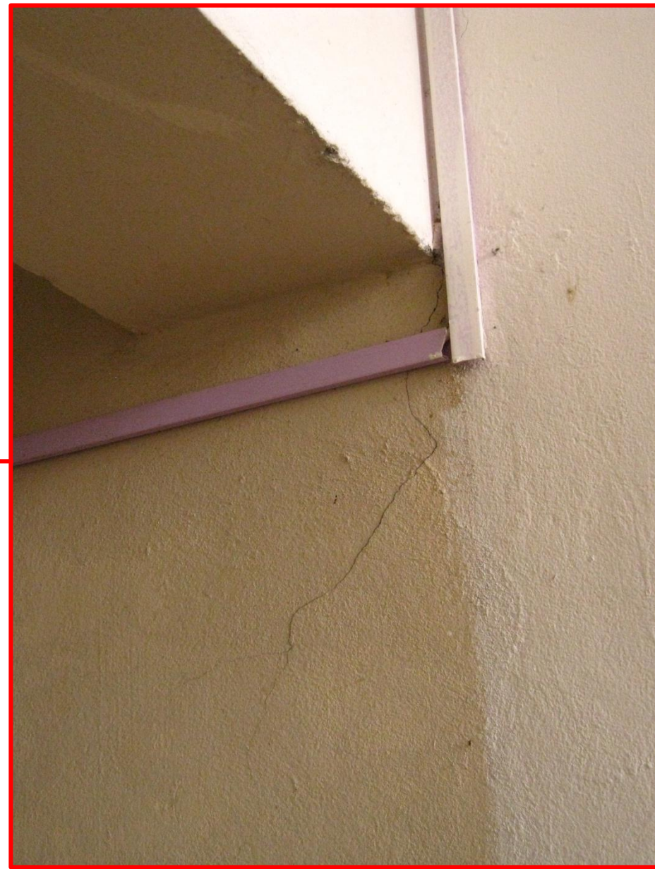
Cracking to masonry wall
