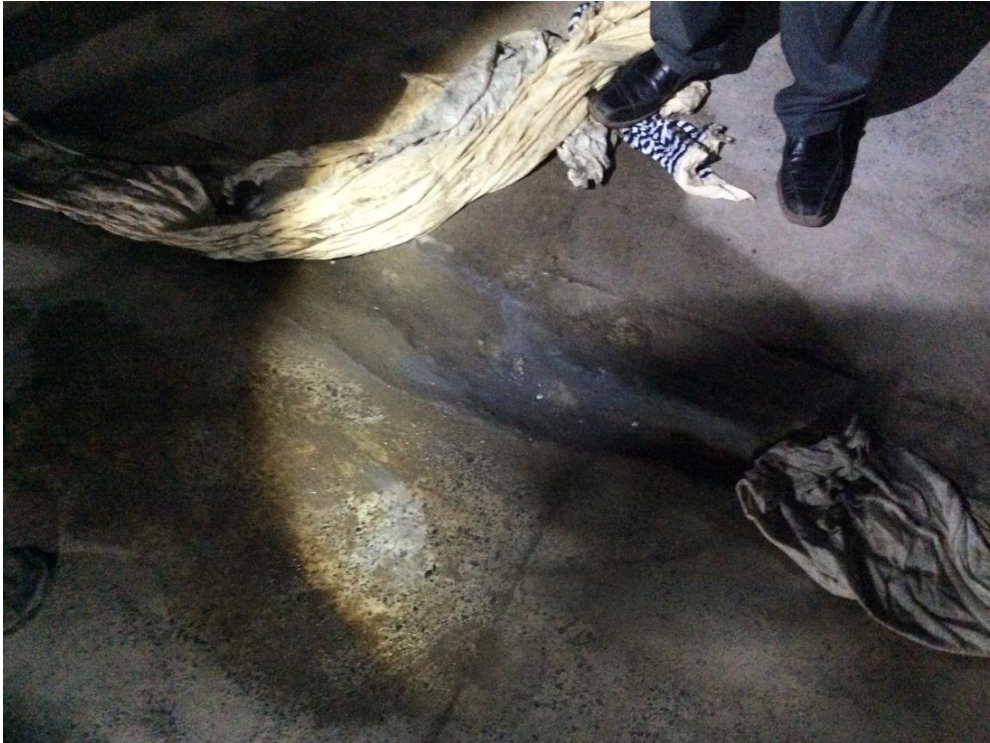
Cracking and water ingress to Basement slab
