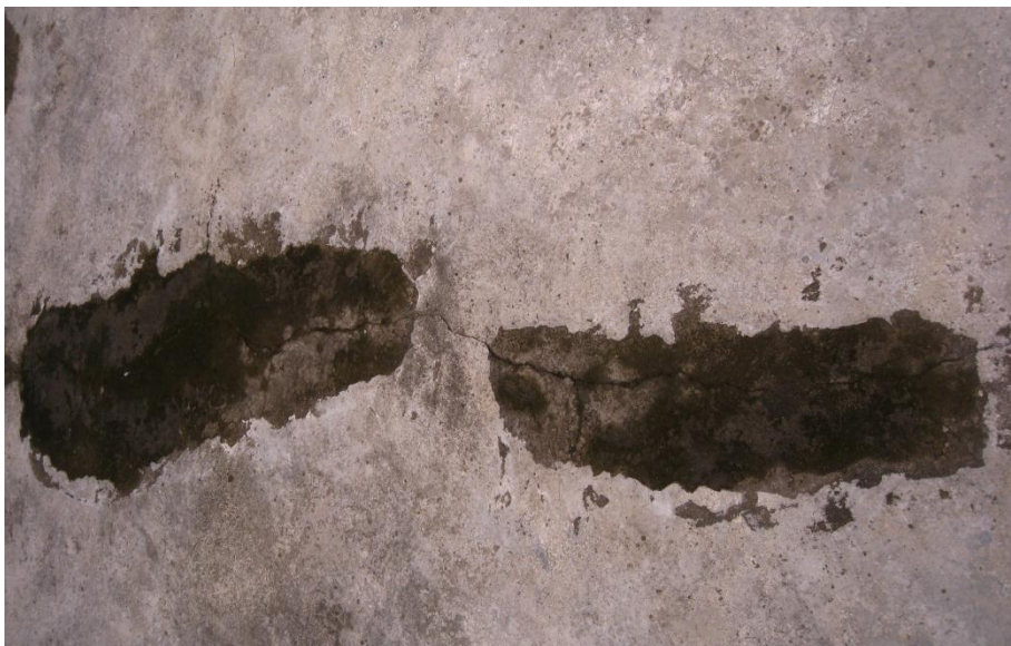
Shed 1 – Cracking to roof slab
