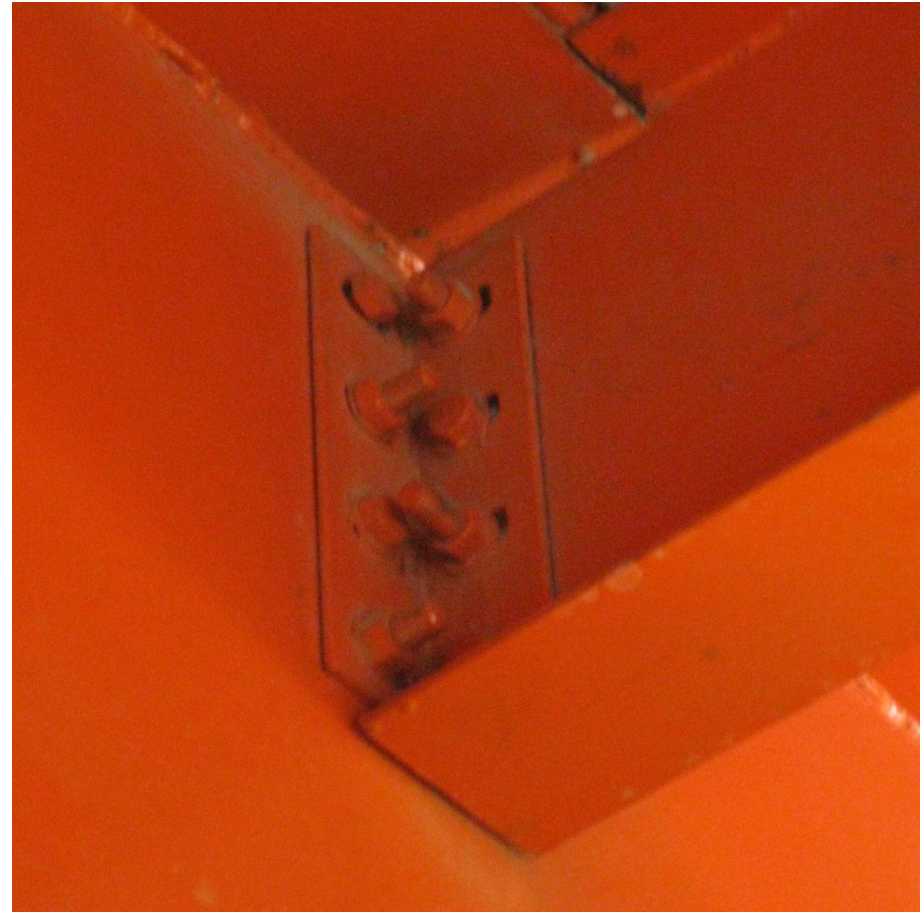
Building 1 – Oversized bolt holes
