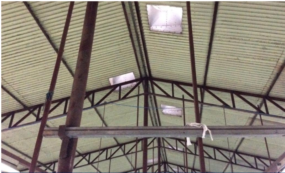
Lateral stability system unclear – no apparent bracing system
