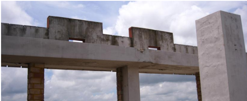
Cracking and deflections to support structure
