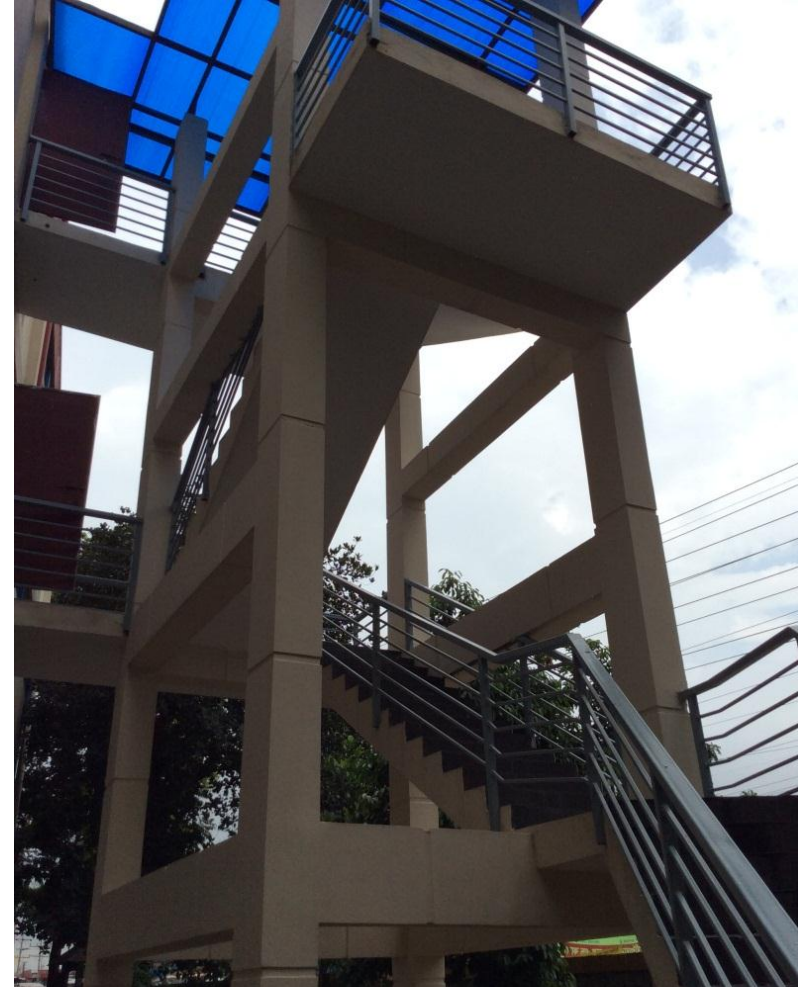
Building 5 – Staircase not shown on drawings
