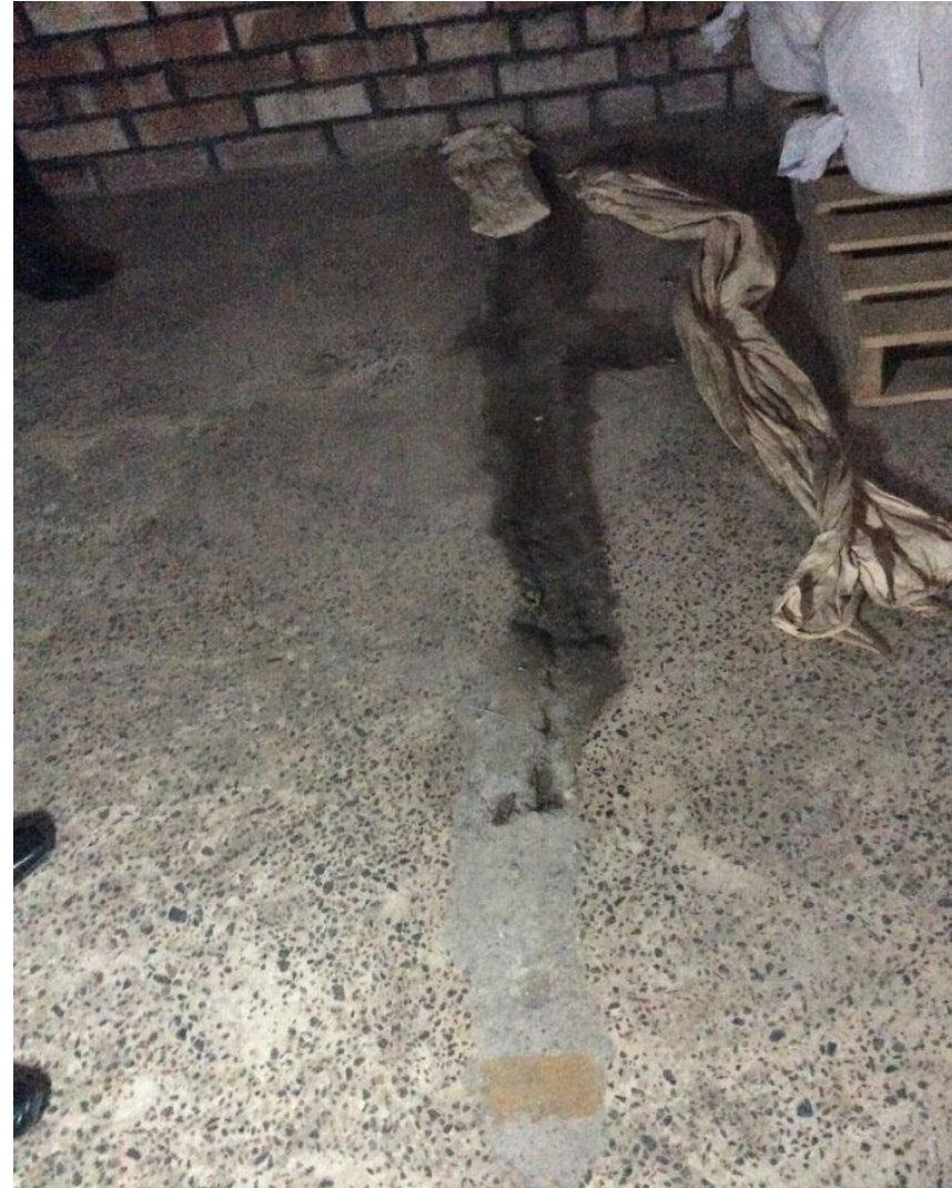
Cracking and water ingress to Basement slab
