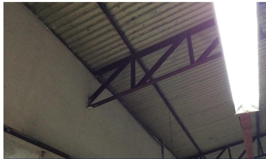
Connection details between trusses and support structure are not clear
