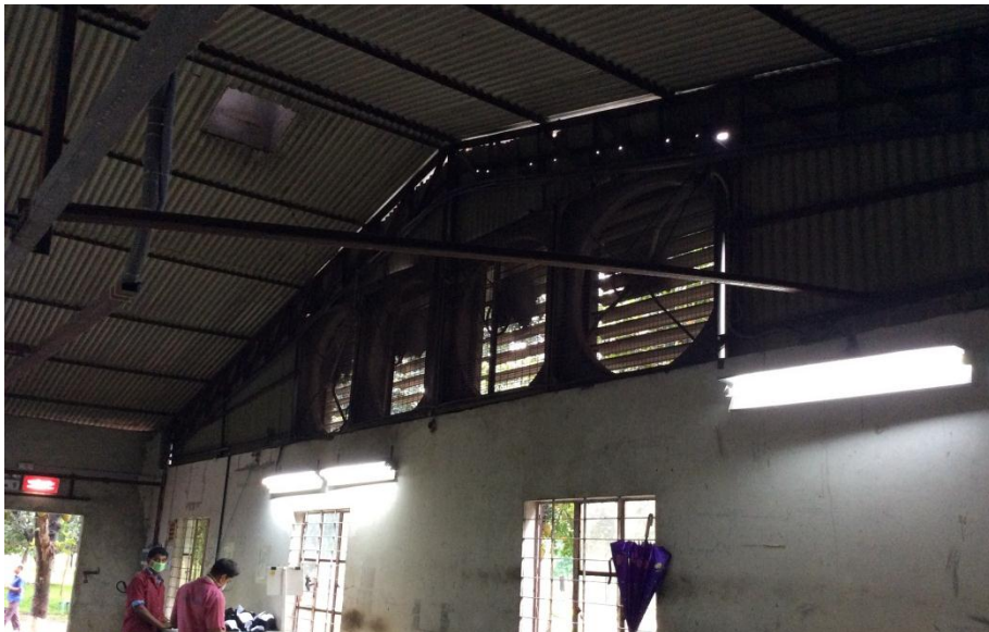
Wind posts missing to gable end
