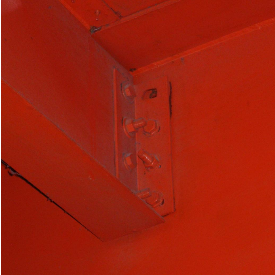
Building 1 – Missing bolts
