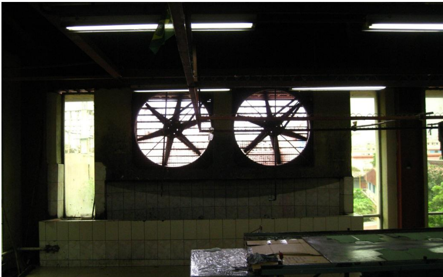
Building 1 – Missing vertical bracing
