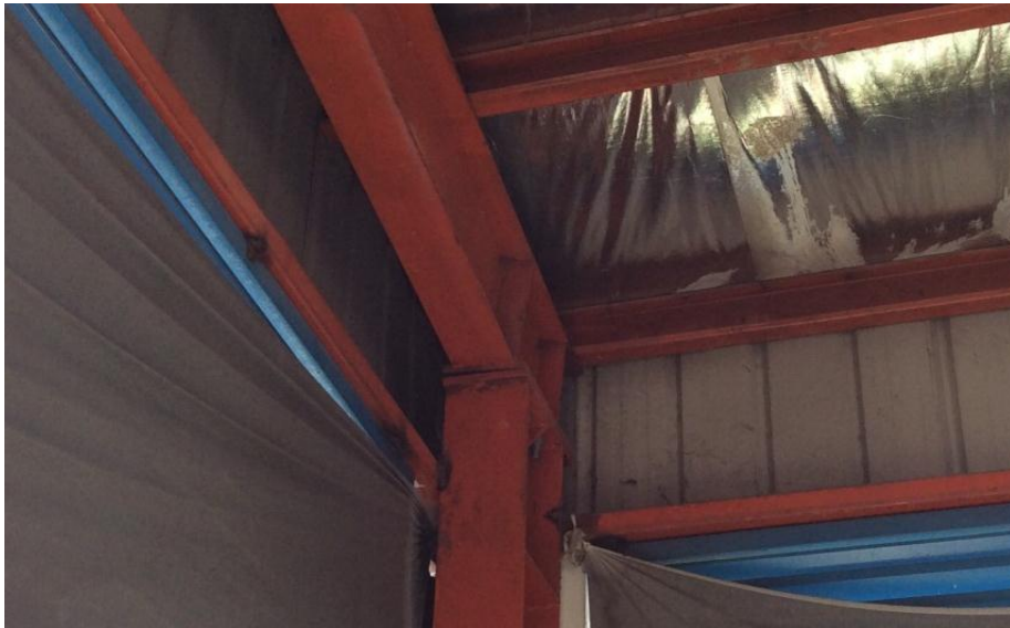
Building 5 – Minimal bearing of end plates
