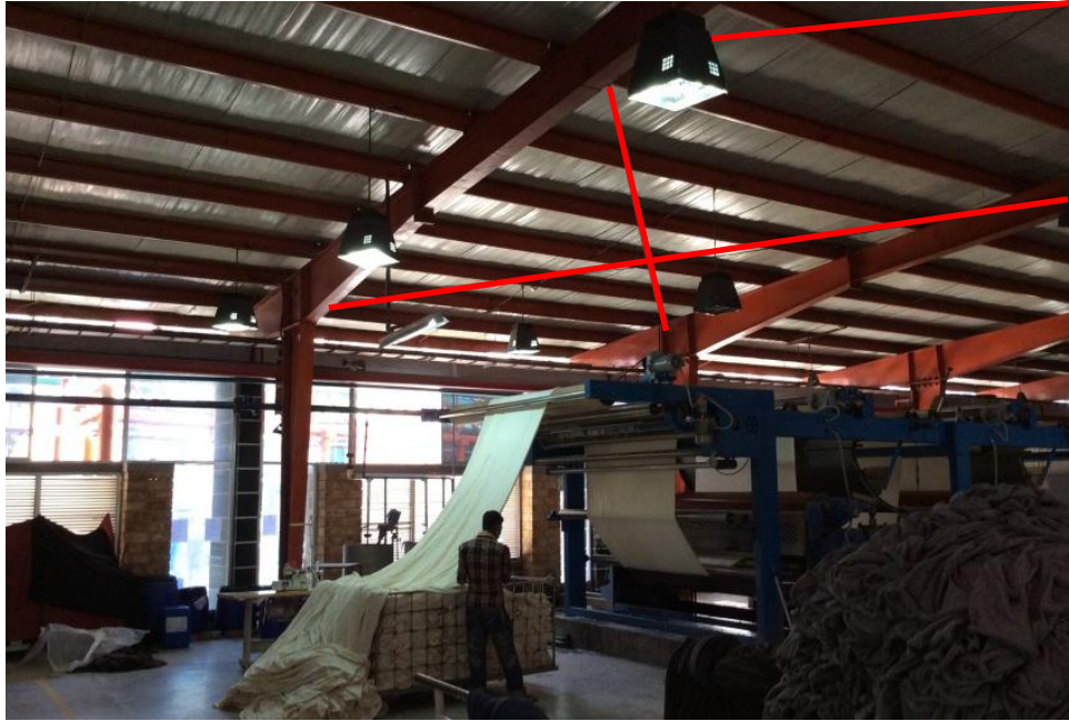
Missing vertical bracing in single storey shed
