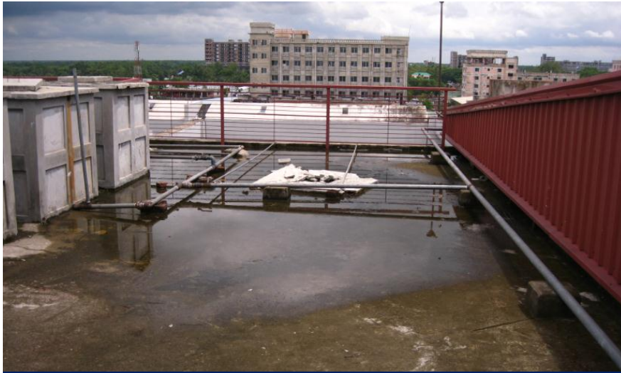
Ponding to roof slab
