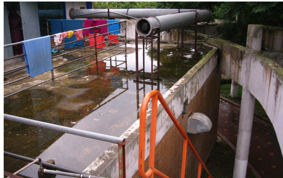
Shed 1 – Water ponding on roof slab
