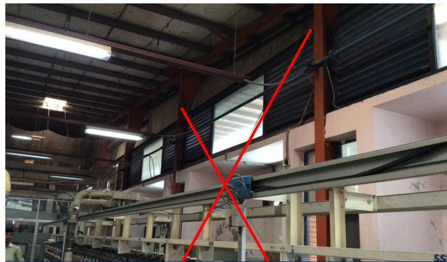
Shed 2 – Bracing not over full height – Building Engineer to review.
