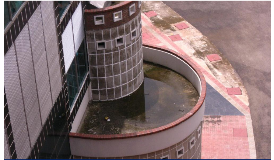
Ponding to roof slab
