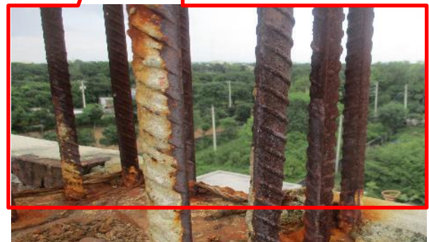
Extensive corrosion was found on exposed rebar
