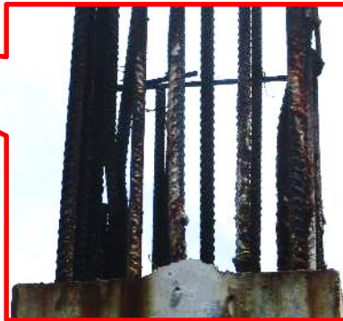
Extensive corrosion was found on exposed rebar
