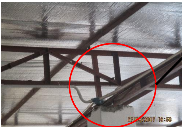
Poor connection detail between RC column and Truss
