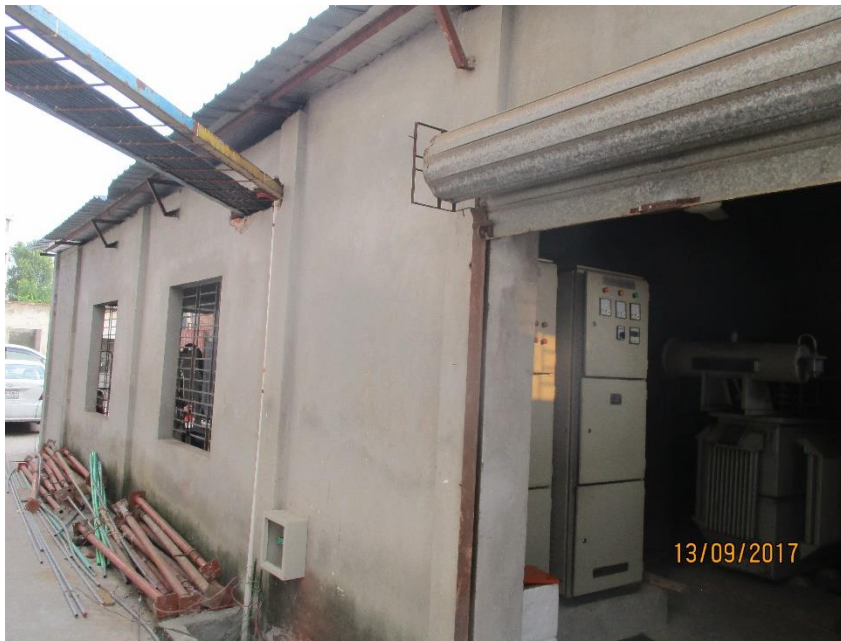
Utility Shed (Generator & Sub-station)
