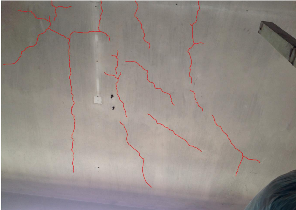
Cracking pattern to concrete slab – u/side 2nd floor
