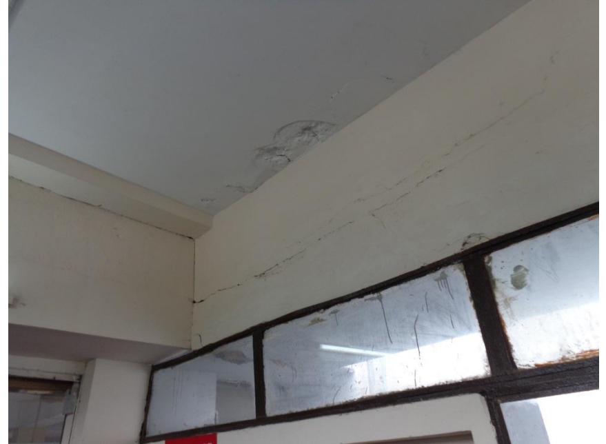
Cracking in masonry and/or concrete lintel causing windows and walls to warp.
