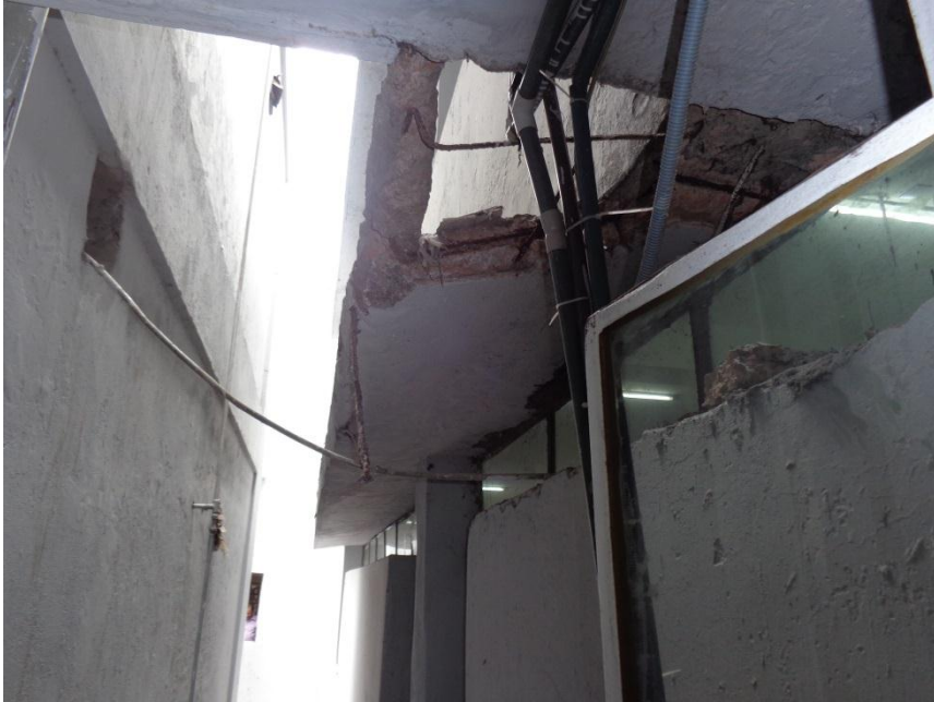
Concrete spalling of awning along exterior corridor wall between adjacent buildings observed at the 1 st and 2 nd storey.
