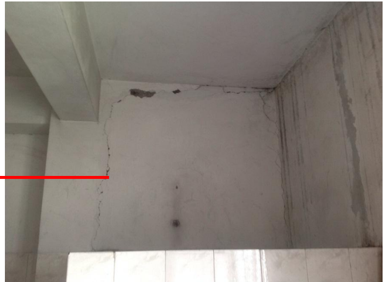
Cracking to 8 th Floor Washroom
