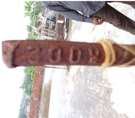
40 not 60 Grade Reinforcing
