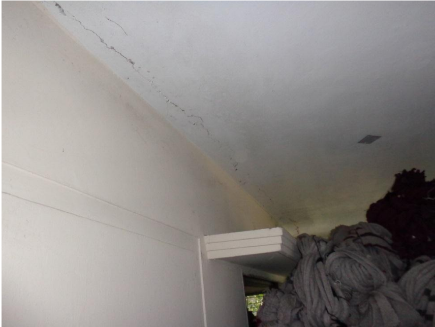
Medium Crack along Joint
