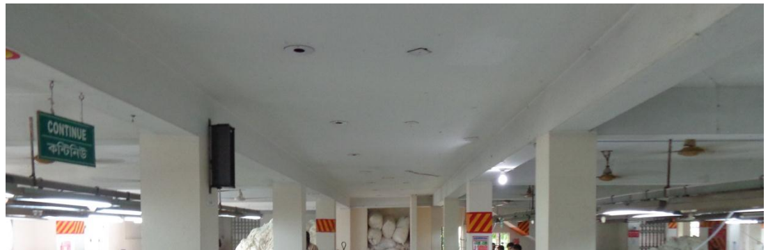
No Beams across Joint
