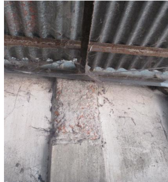
Connection between steel angle and RC column was not clear
