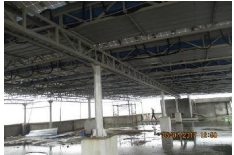
Apparently lack of lateral stability system observed on truss supported Solar panel.
