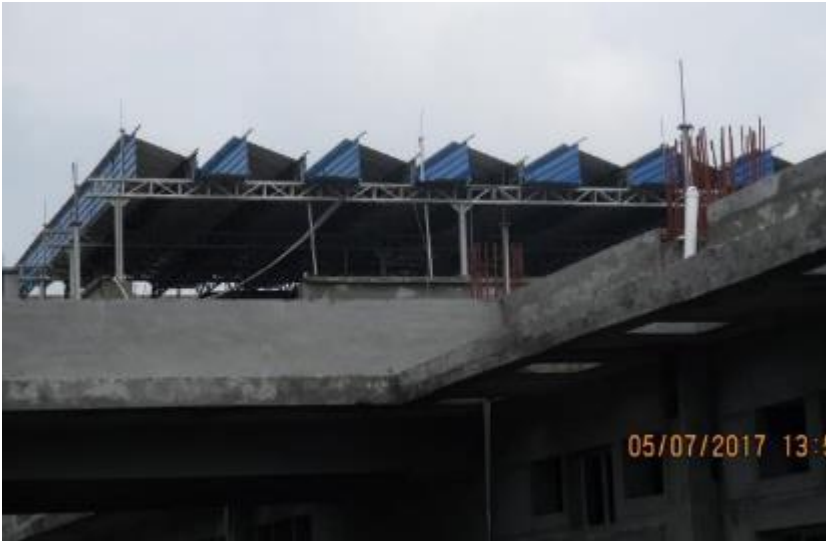
Roof top Solar panel
