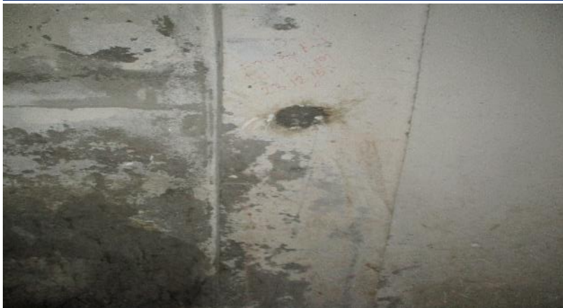
Dampness observed on Peripheral Wall
