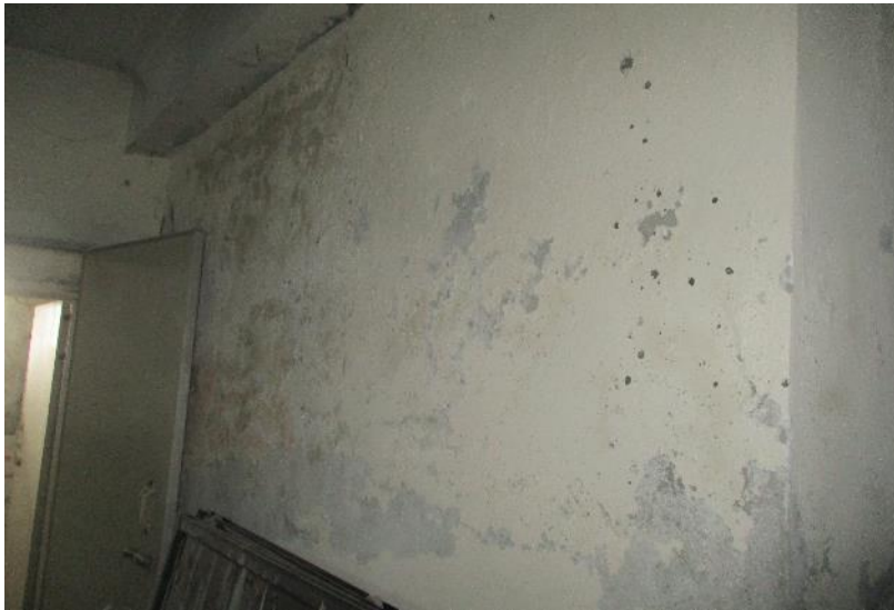
Dampness observed on wall beside toilet area.
