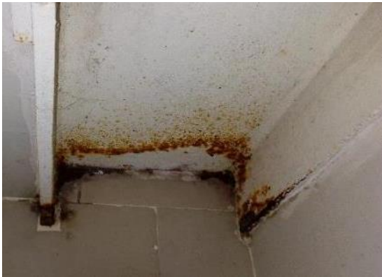
Corrosion at steel column
