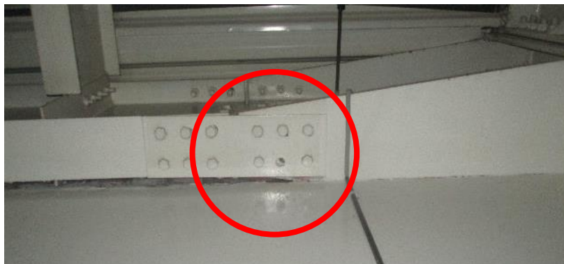
Bolt missing at joint of Main Beam
