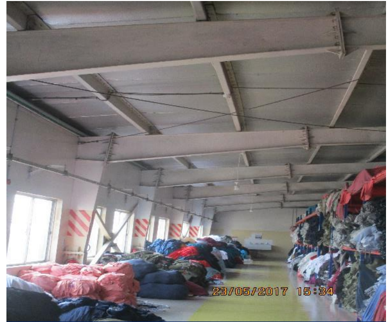
Loose horizontal bracing observed at roof shed of the factory building
