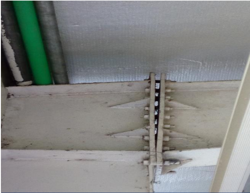
Loose connection between rafters
