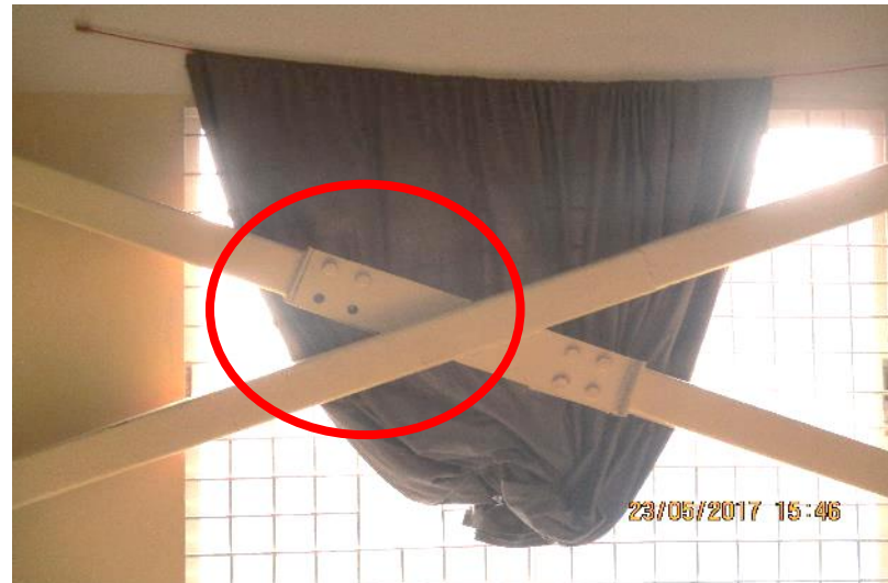
Bolt missing of bracing at 4 th floor
