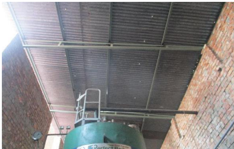
Non engineered roof shed of boiler
