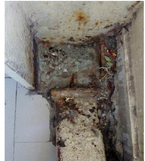
Corrosion at joint
