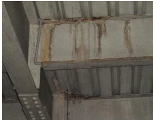
Corrosion at Sub Beam
