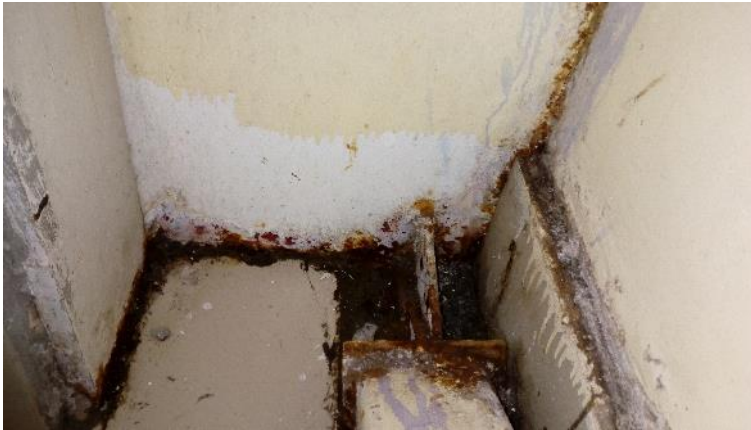
Corrosion at joint
