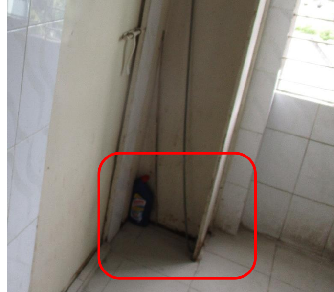
Corrosion at column base inside toilet zone
