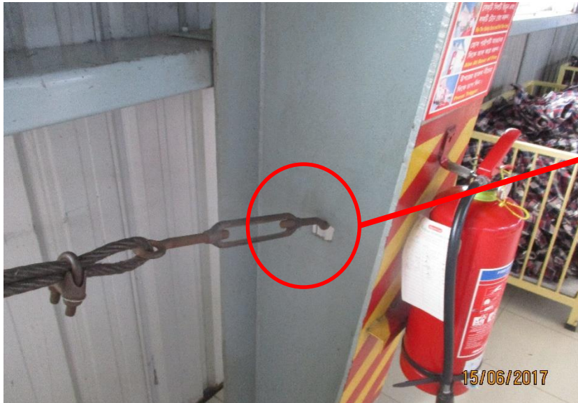
Poor bracing connection
