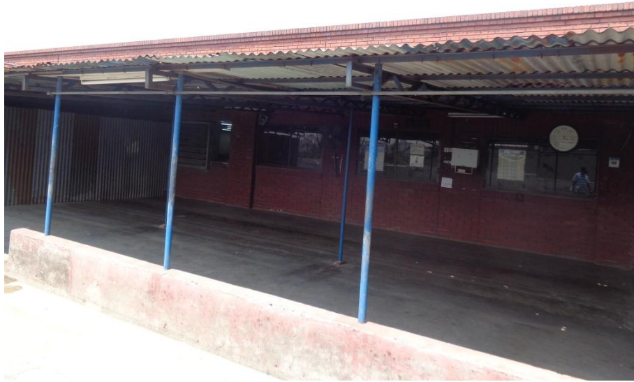
Poor truss to column connection for steel roof of main building
