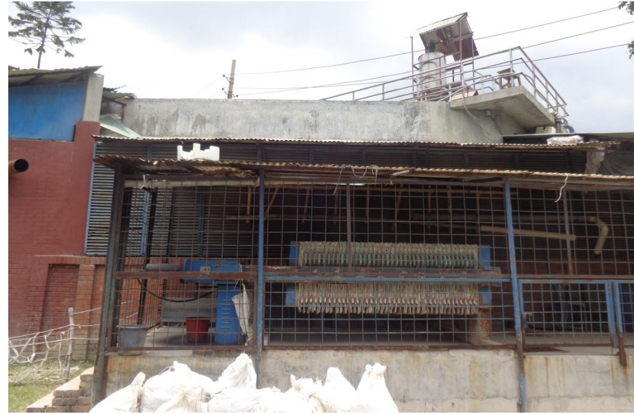
Poor corrugated steel and purlin detailing at ancillary sheds
