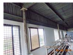
Figure: Corrosion in steel column
