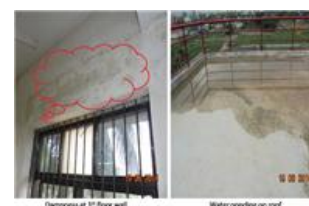
Dampness at 1 st floor wall Water ponding on roof Figure: Presence of dampness and water ponding
