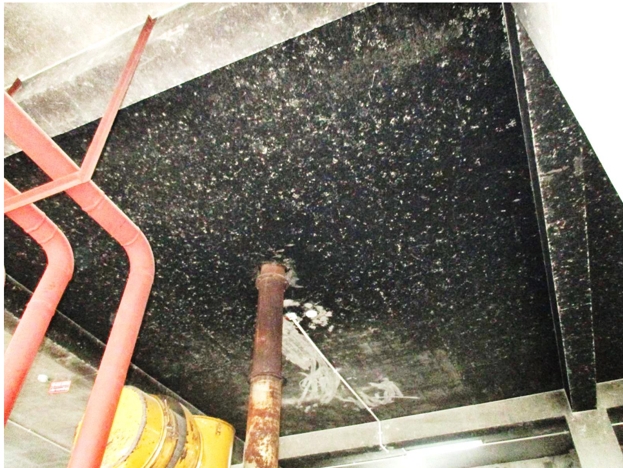
Carbonation was observed in the soffit of slab
