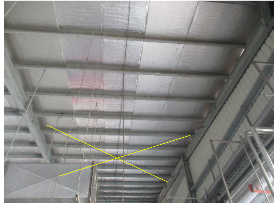
At south roof bracing does not continuous to end. Bracings are shown yellow in picture.
