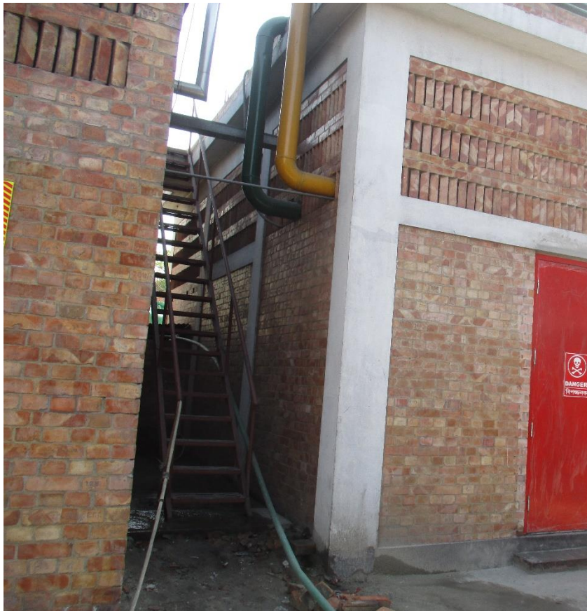
External steel stair between Boiler & Chiller room
