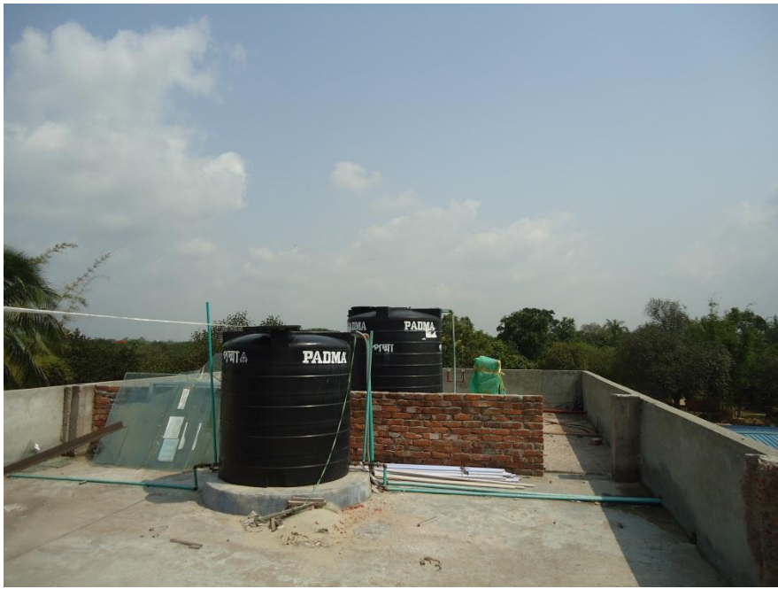
Roof level of Building 2 (the only non-steel roof on the site), with no waterproofing present.
