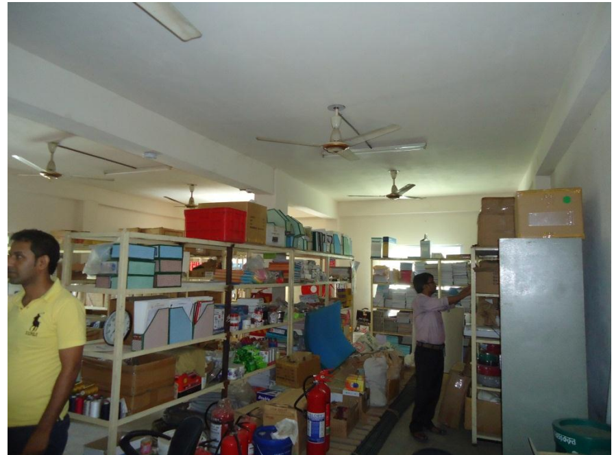
View from inside Building 2, at 1 st floor level. As this image shows, no signs of water ingress were evident.
