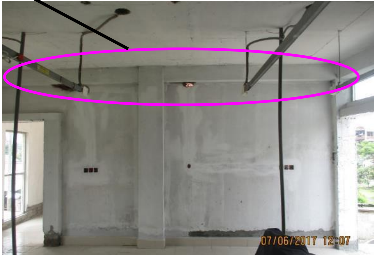
Depth of stair case beam was found 1 inch less then provided drawing
