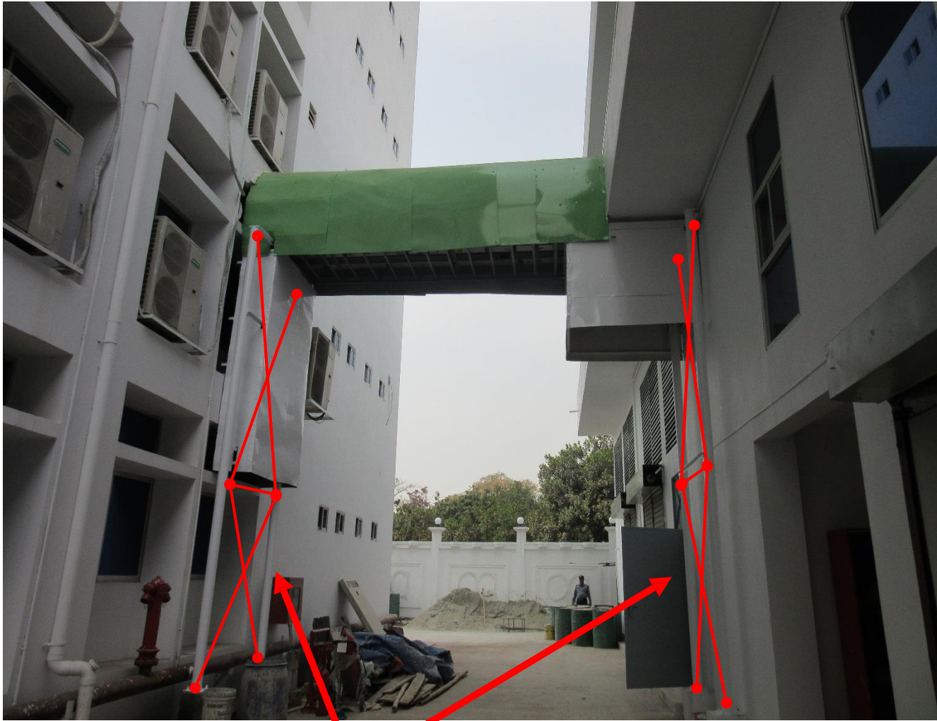
Lack of stability bracing
