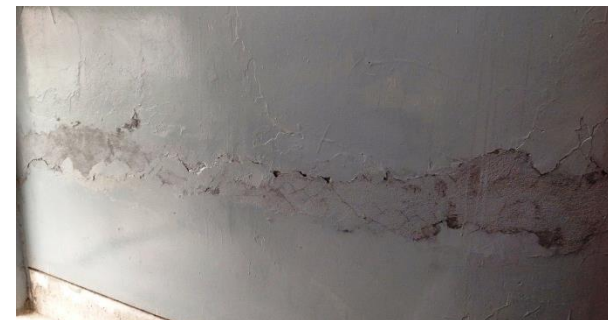
Building 2 – Cracking to SE stair wall
