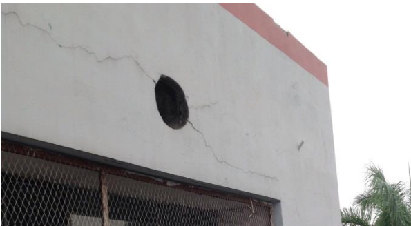
Building 2 - Cracking to SE corner
