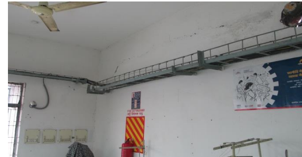
Building 2 - Cracking to NE corner
