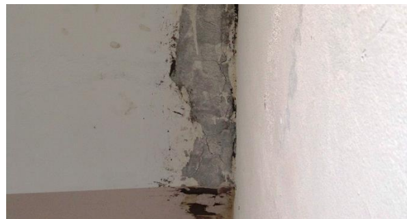
Building 2 – Cracking to SE stair slab
