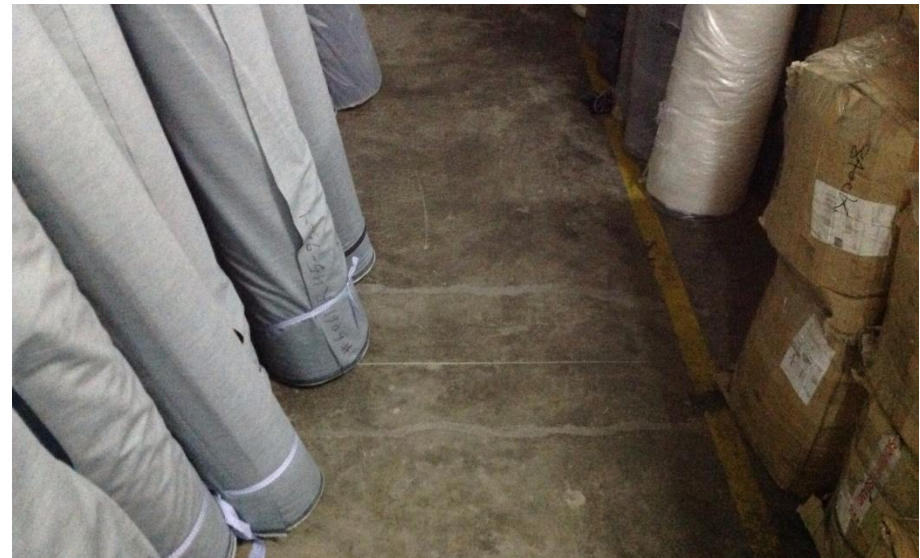
Building 2 – Cracking of slab along beam lines at 1 st Floor
