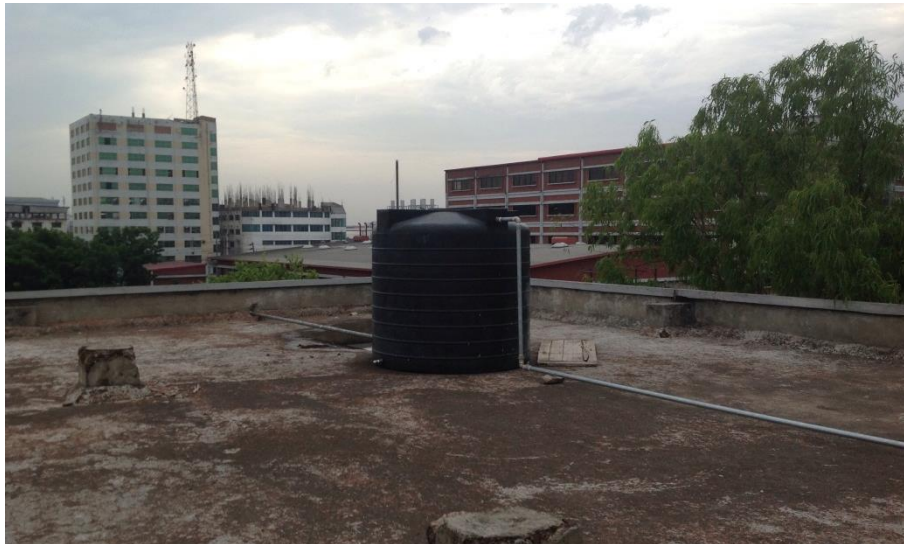
Building 1 – 5000 litre water tank at Roof Level
