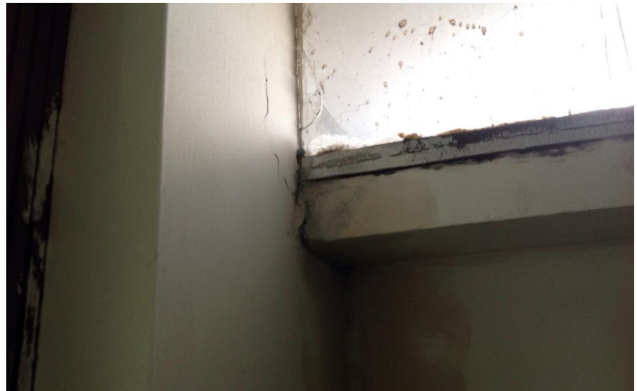
Cracking and evidence of remedial works to Building 2
