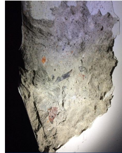
Tested Ground Floor Column – Stone Chips
