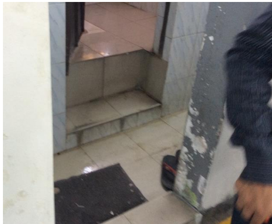
Build up on toilet floors
