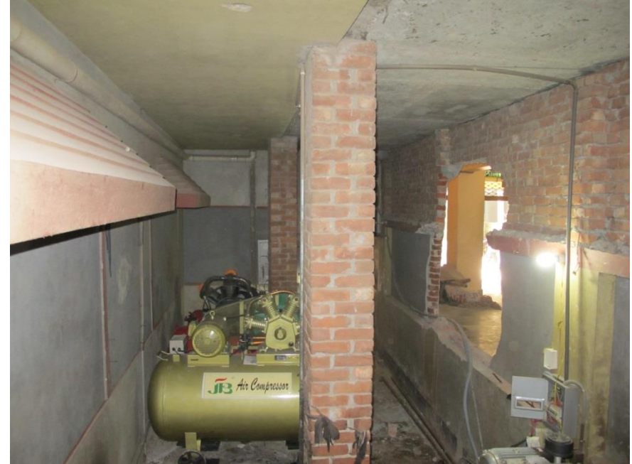
Masonry columns at ground floor apparently centred on movement joint
