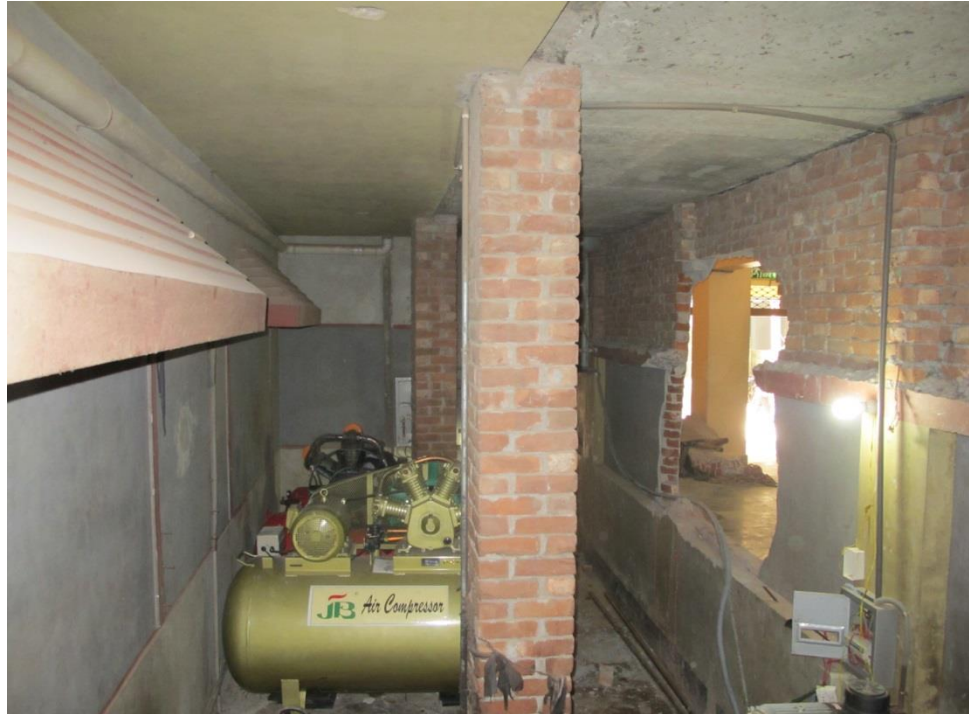
Purpose of masonry columns not apparent.
