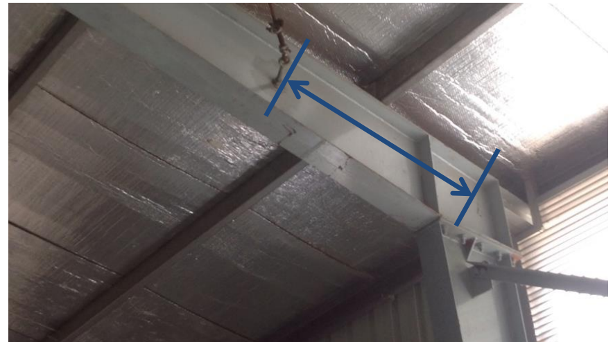
Plan bracing substantially away from vertical supports
