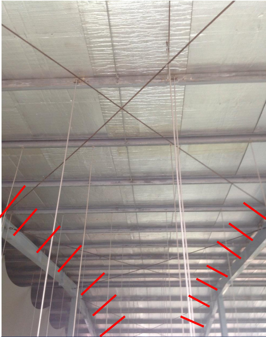
Missing compression flange braces
