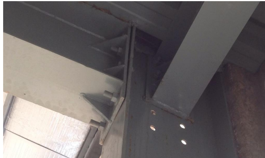
Gaps to connections
