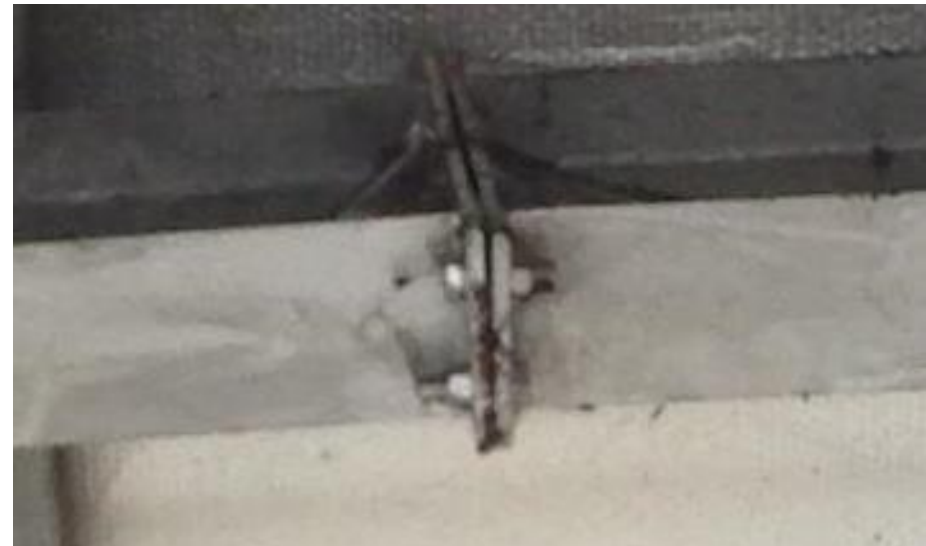
Gaps to connections
