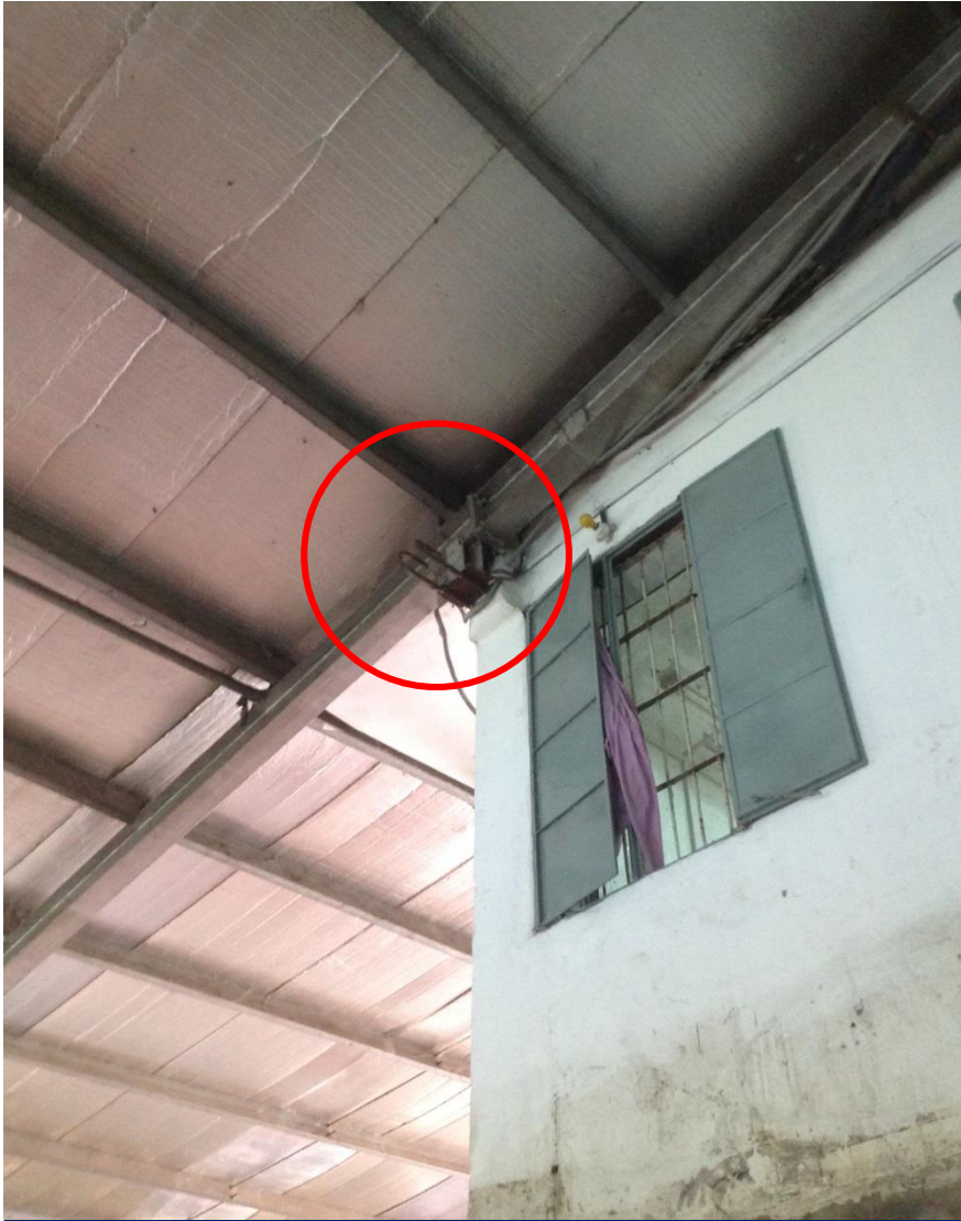
Capacity of support points of portal frame unclear.
