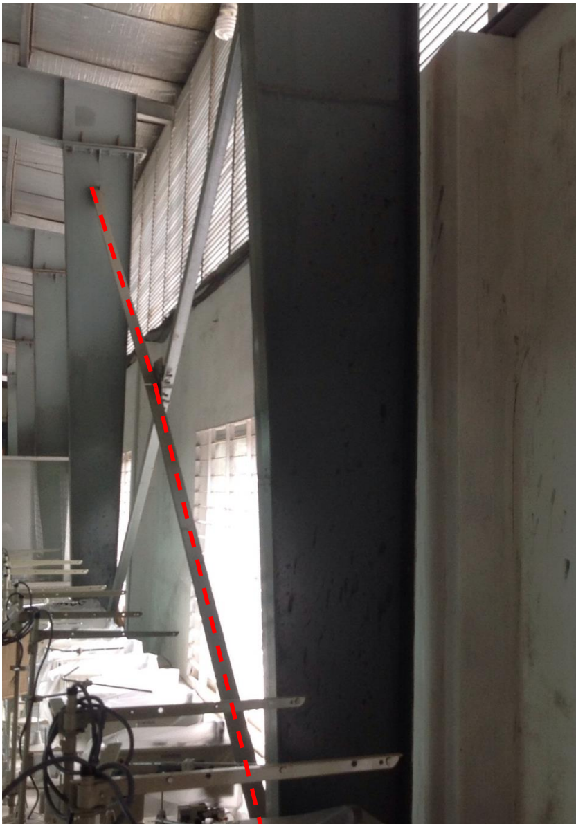
Untightened vertical braces
