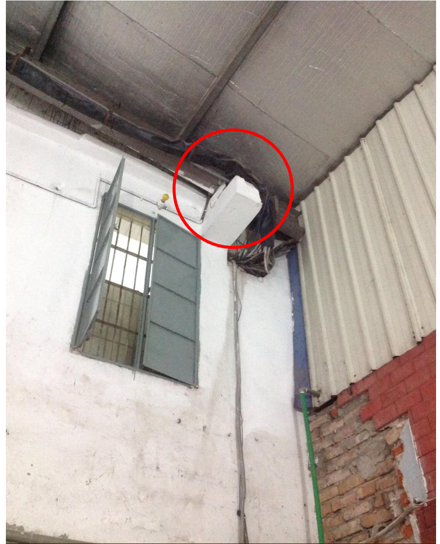
Support points of portal frame unclear.
